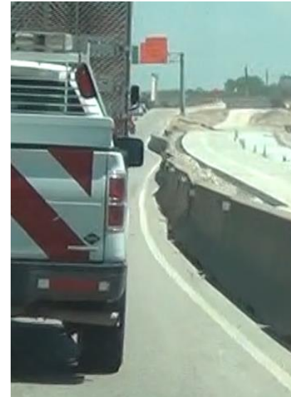
Figure 1. Barrier Creep with Unanchored Temporary Barriers in Freeway Work Zones.
