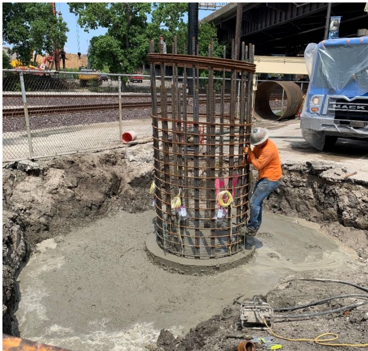
Figure 4-19: Concrete for Ramp F Bent 5 drilled shaft is over-poured.
