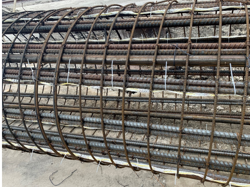
Figure 4-7: Conventional TIP wires affixed to the reinforcing cage for the Ramp F Bent 6 drilled shaft.
