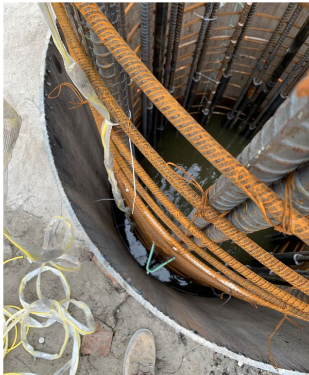
Figure 4-8: Conventional TIP wires affixed to the outside of the reinforcing cage for the Ramp F Bent 6 drilled shaft.
