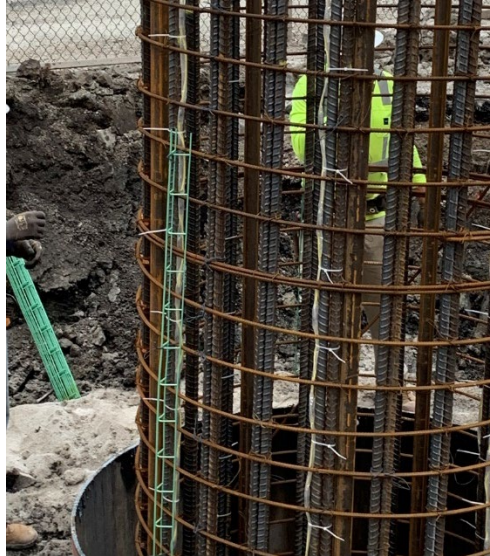
Figure 4-13: Reinforcing steel chairs used as centralizers for the Ramp F Bent 5 drilled shaft.
