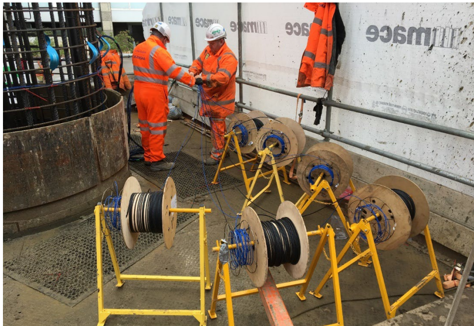
Figure 2-6: Distributed fiber optic sensing cable installation for a drilled shaft in the United Kingdom.
