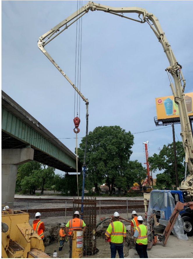
Figure 4-18: Placement of concrete by tremie in the drilled shaft for Ramp F Bent 5.
