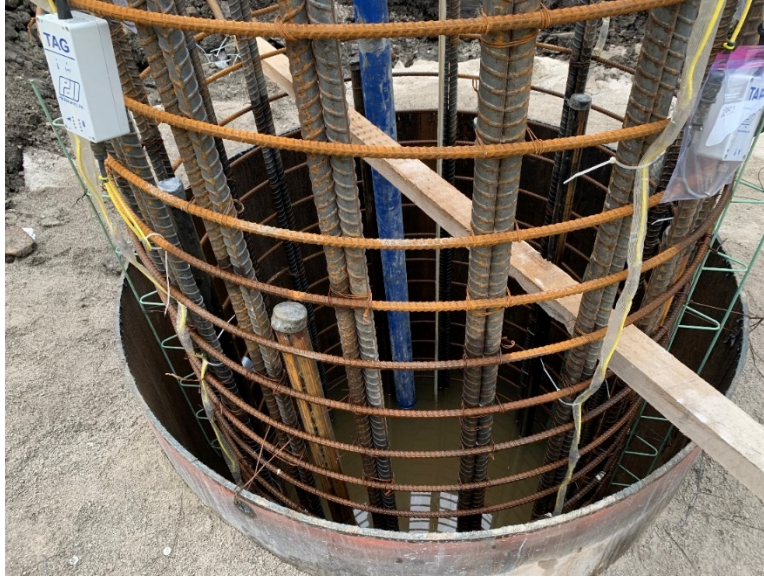
Figure 4-21: TIP wires connecting into a TAG box (left) and TAP box (right). The boxes are attached to the top of the reinforcing cage for the Ramp F Bent 5 drilled shaft.
