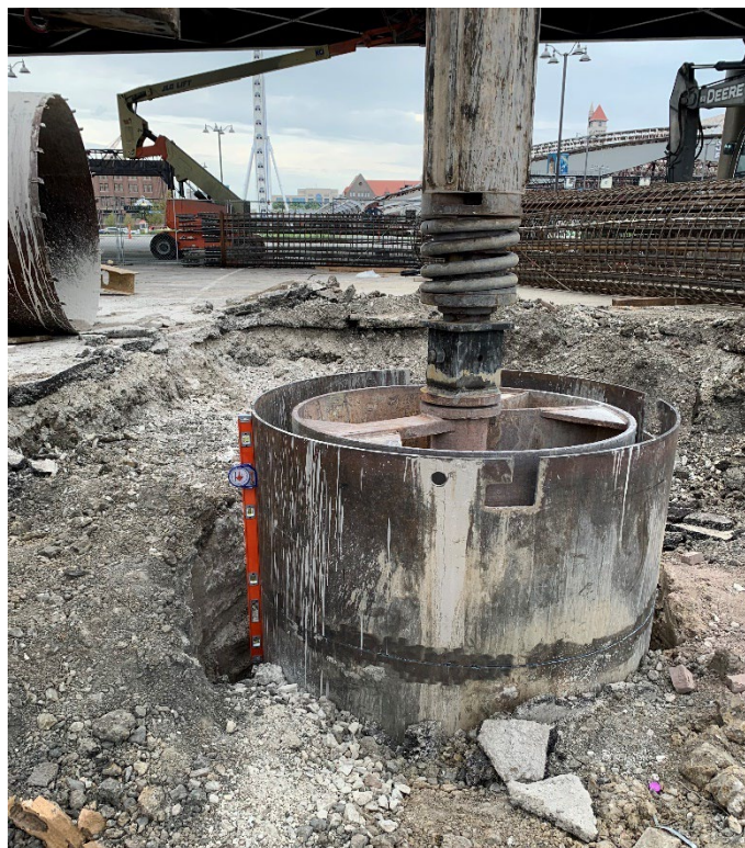
Figure 4-6: Ramp F Bent 6 shaft after welding an extension piece to the top of the permanent casing. In this photo, the temporary casings have been removed and the ground near the shaft has been excavated to provide a safe working space for reinforcing cage and concrete placement.
