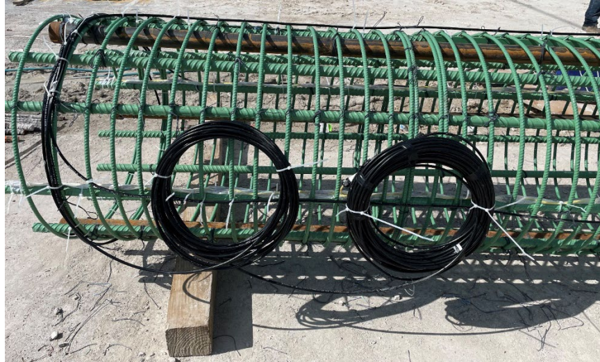
Figure 4-10: Thermal fiber optic cables pre-installed on bottom section of reinforcement cage, with bundles for final vertical attached to the side of the cage.
