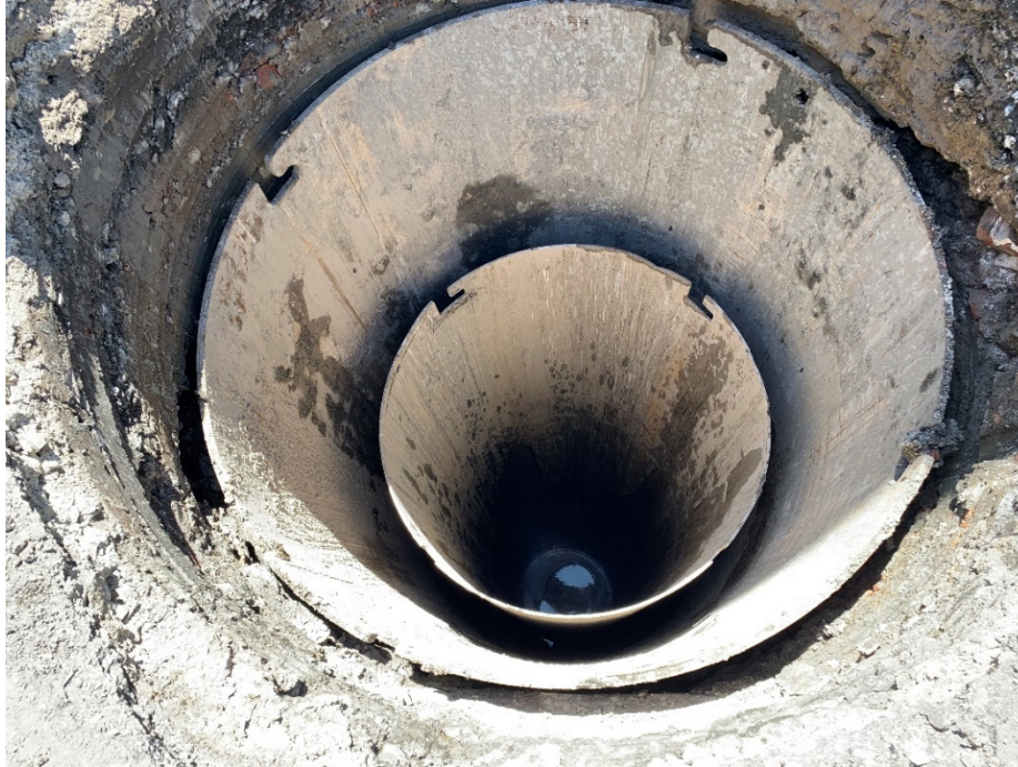
Figure 4-5: Excavated shaft for Ramp F Bent 6 with the permanent (innermost) 72-inch casing and temporary 84-inch casing shown.
