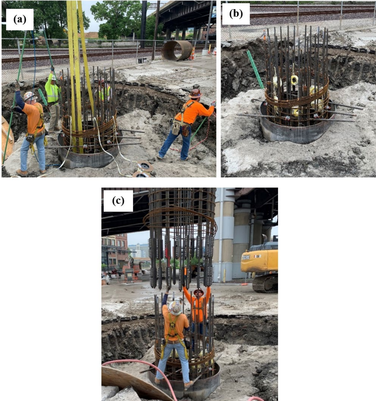
Figure 4-12: Reinforcing cage placement for the Ramp F Bent 5 drilled shaft: (a) lower half of cage suspended with the crane, (b) lower half of cage resting on casing, and (c) top half of cage aligned with bottom half prior to engaging mechanical bar splices.
