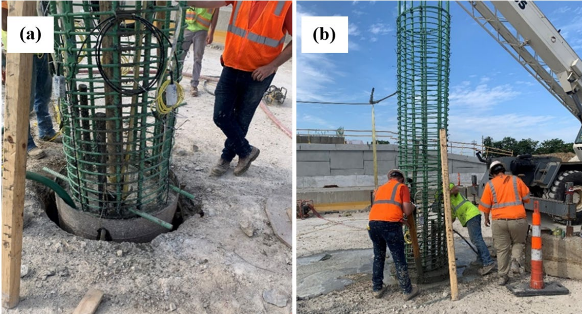
Figure 4-16: Concrete placement for Ewing Shaft 3: (a) Gap between the outside of the permanent casing and the ground surface; (b) overpouring concrete at the end of placement.
