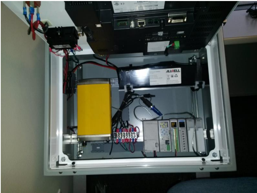
Figure 62. First version of PLC system hardware (battery, PLC, terminal strip, and GPS unit shown with HMI panel raised).
