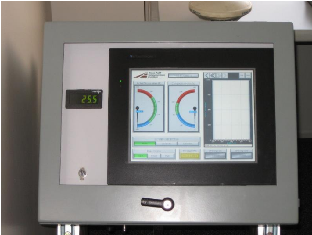
Figure 61. First version of PLC system hardware (main HMI screen shown).
