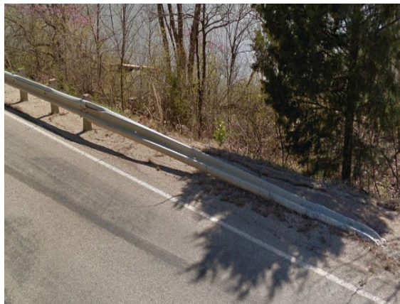
Figure 2.18: Turndown End in the Field
