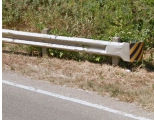
Figure 2.16: Breakaway Cable Terminal in the Field
