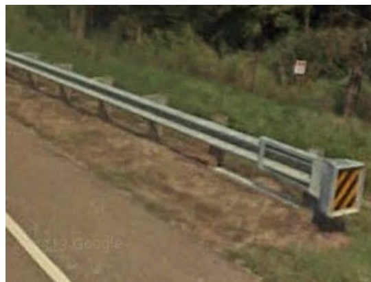
Figure 2.15: Energy-Absorbing Guardrail End in the Field
