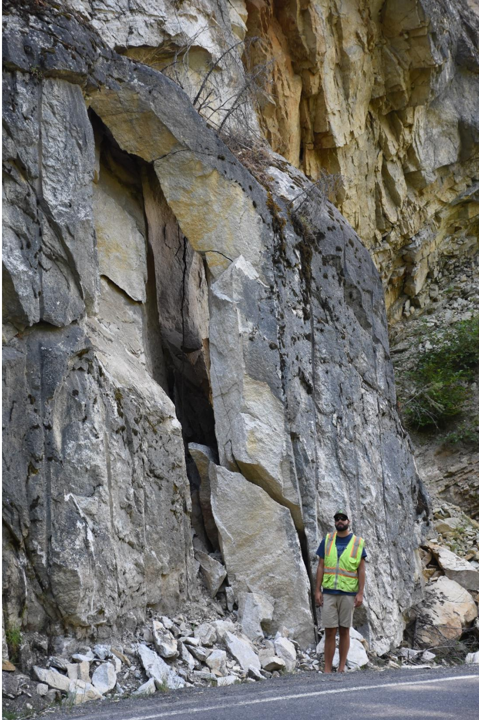
Figure 3.6 Photograph of a rockfall along SH-14 west of Elk City (45.811995°, -115.631704°E).
