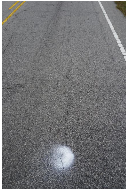
Figure 22. Cracks on NC 96 pavement surface.
