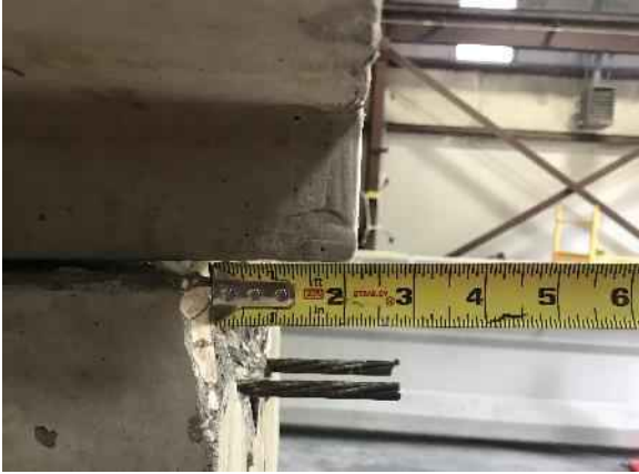
Figure 10-17 Horizontal interface displacement (Girder A2_1)
