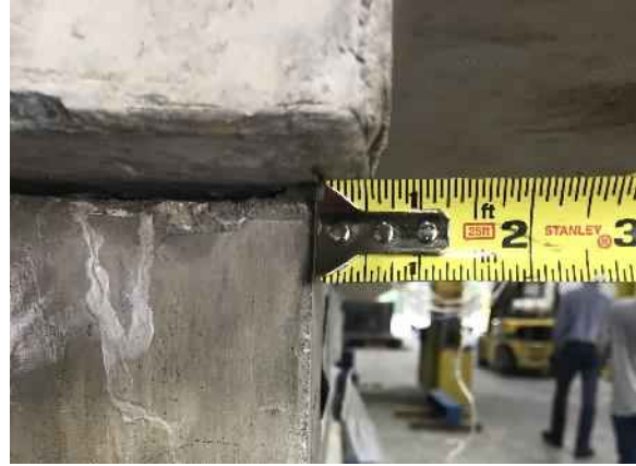
Figure 10-18 Horizontal interface displacement (Girder A2_2)
