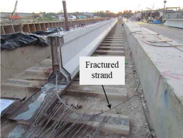
Figure 4-17 Bed end after breakage of the HSSS strand
