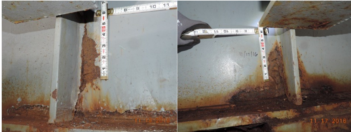
Figure 10: Vertical and Horizontal Fatigue Cracks on the Left Side of the Web Stiffener
