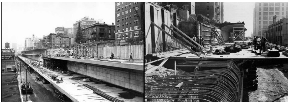
Figure 12: Brooklyn-Queens Bridge Triple Cantilever Picture During Construction (Reference: New York City Parks Photo Archive)
