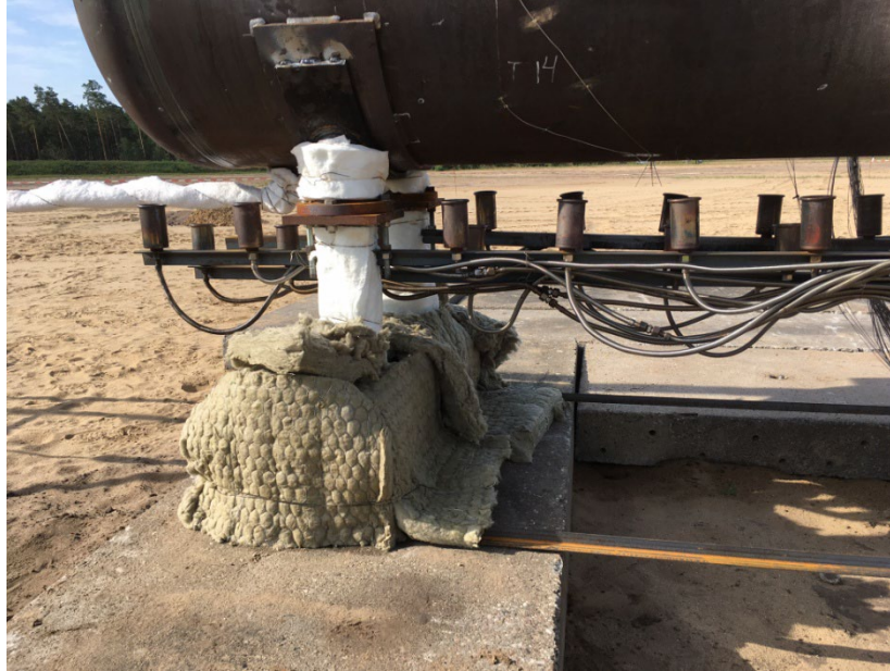
Figure 17. Support legs and water bath with insulation
