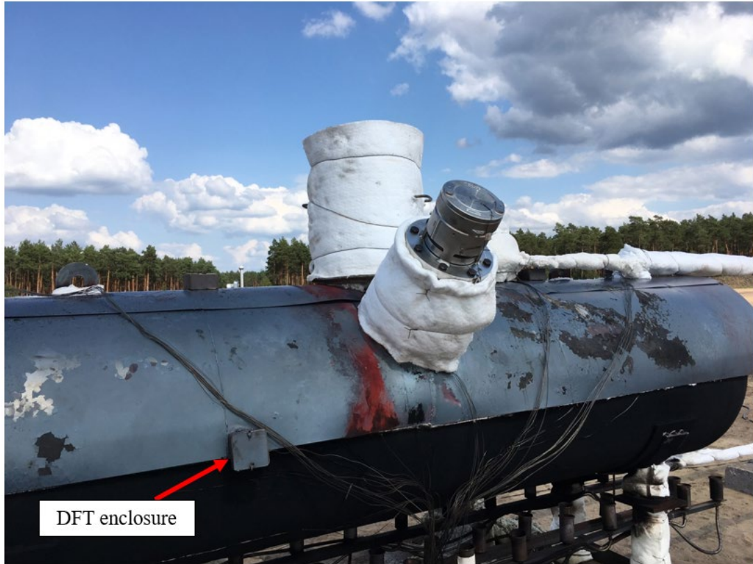
Figure 18. Nozzles with insulation and large capacity PRD at 45 degree orientation
