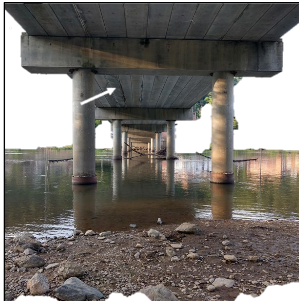
Figure 13. The white arrow points to one of several parallel crevices in MB over the French Broad River in western North Carolina where gray bats were visible through binoculars and with the aid of a 1,000-lumen spotlight from the underside of the bridge.
