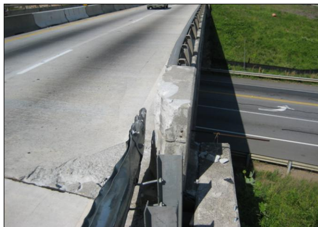
Figure 5.16 Issues with clearance on bridges
