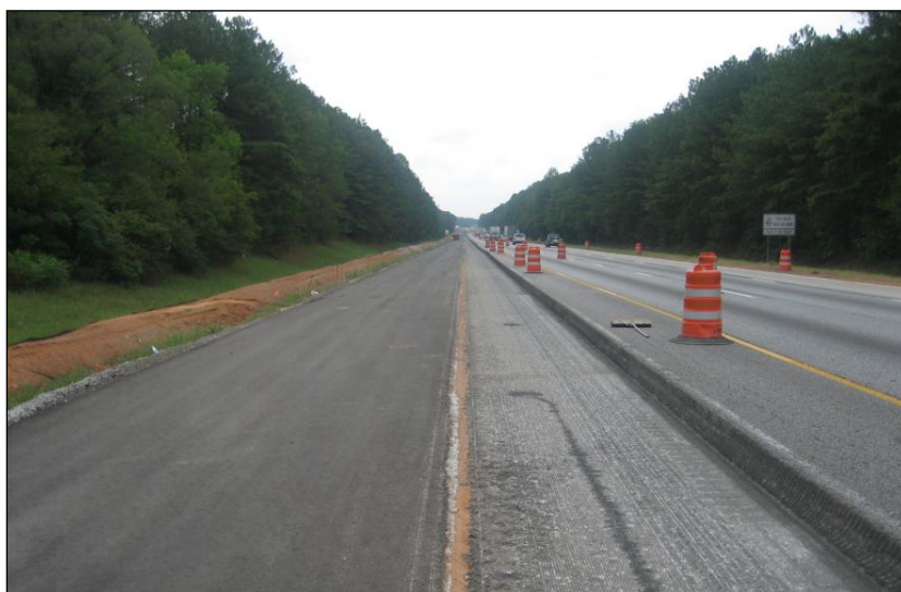
Figure 5.13 Insufficient asphalt base under travel lanes
