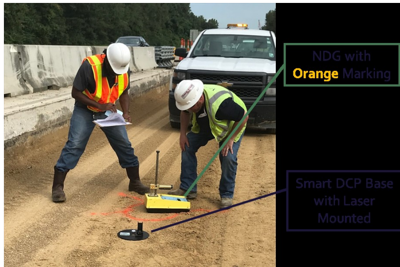
Figure 14. I-10 Zone 124 NDG and Smart DCP setup
