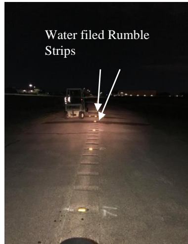
Visibility of water-filled rumble inserts (100 ft)
