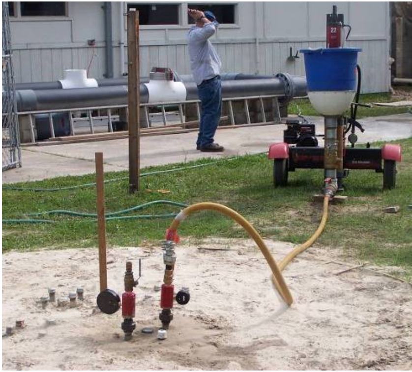
Figure 4-22 The 1.5-inch high pressure line connected from the grout pump to the pile.
