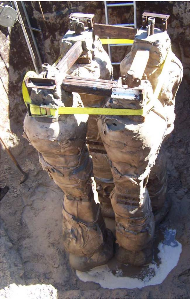
Figure 4-33 Exposed pile group.
