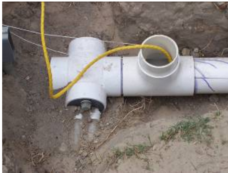
Figure 4-9 Pipe system for routing stress gage wiring to monitor facility.
