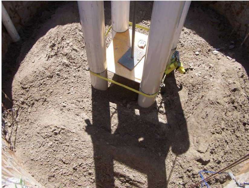
Figure 5-4 Filling the test chamber.
