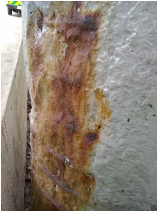
Figure C 14 - DEL 71 498 center column SB over spall
