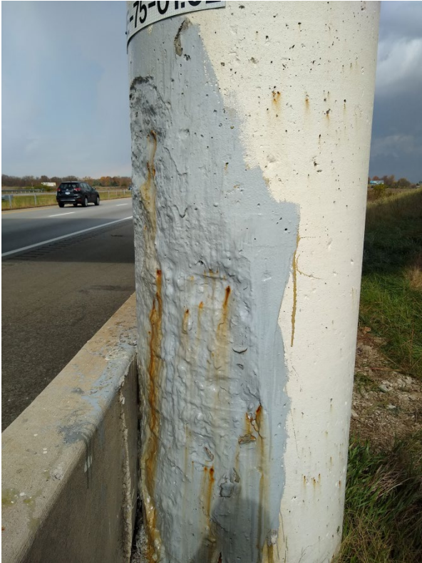
Figure C 28 - - SHE 75-0102 coating failure
