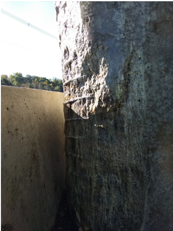
Figure C 3 - - Spalled area on center SB column
