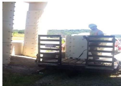
Figure A 5 - Assembled shield nested on trailer
