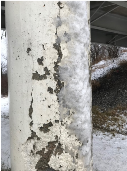
Figure 1 - Pier column with snow thrown from a plow. (Courtesy D. Wise, ODOT)
