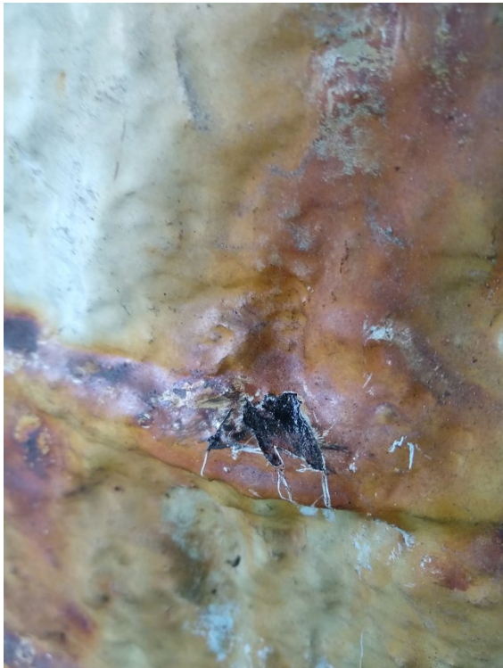
Figure C 18 - DEL 71-1093 V notch over spall on center SB column.
