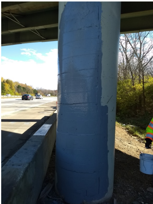
Figure C 7- Patch on FRA 270 960 coated with Citadel product
