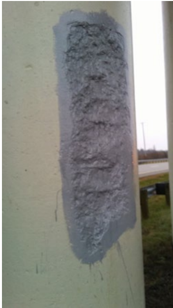
Figure C 19 - Spall on MIA 75 1995
