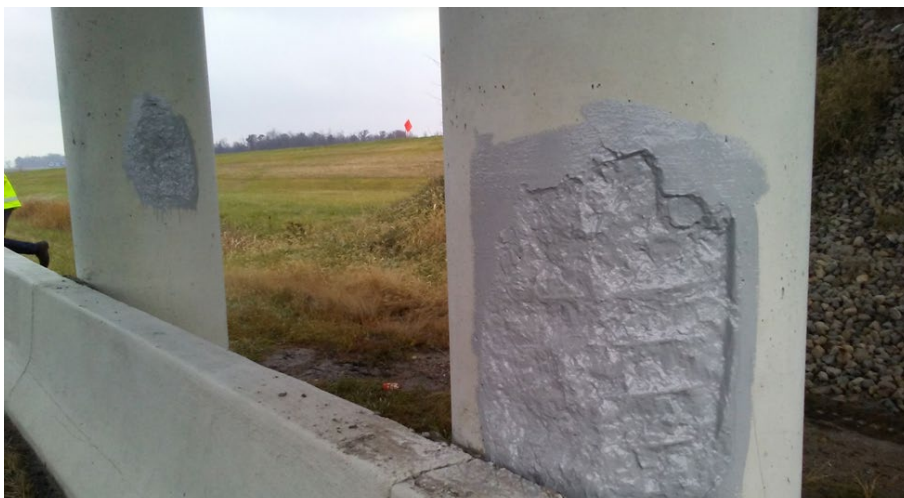
Figure C 21 - Spalls on SHE 75 1954
