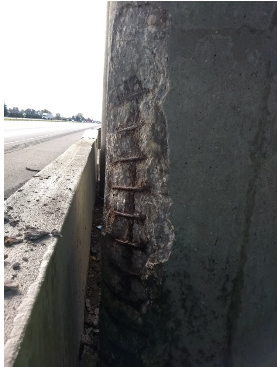
Figure C 5 - Spall on center SB column DEL 71-1093
