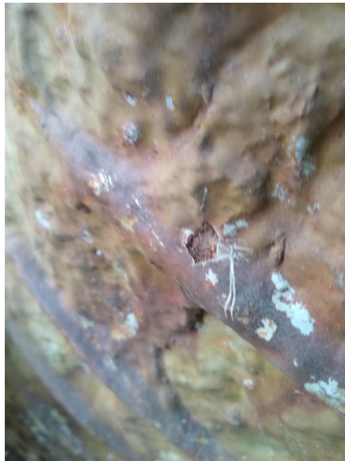
Figure C 15 - DEL 71 498 V notch center column SB at spall.
