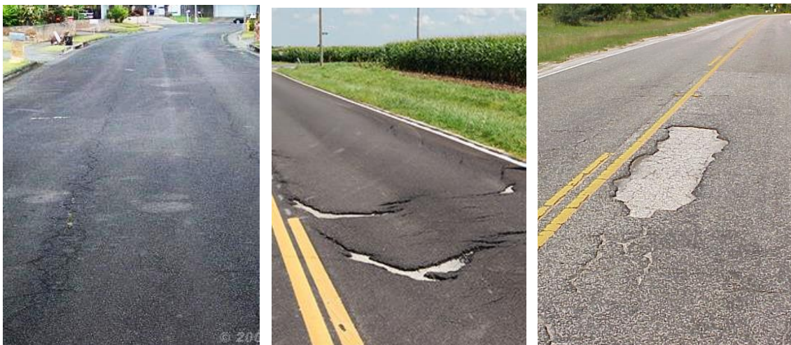
Figure C.1: Distresses Associated with Poor Bonding: (a) Fatigue Cracking, (b) Slippage Failure, and (c) Delamination.
