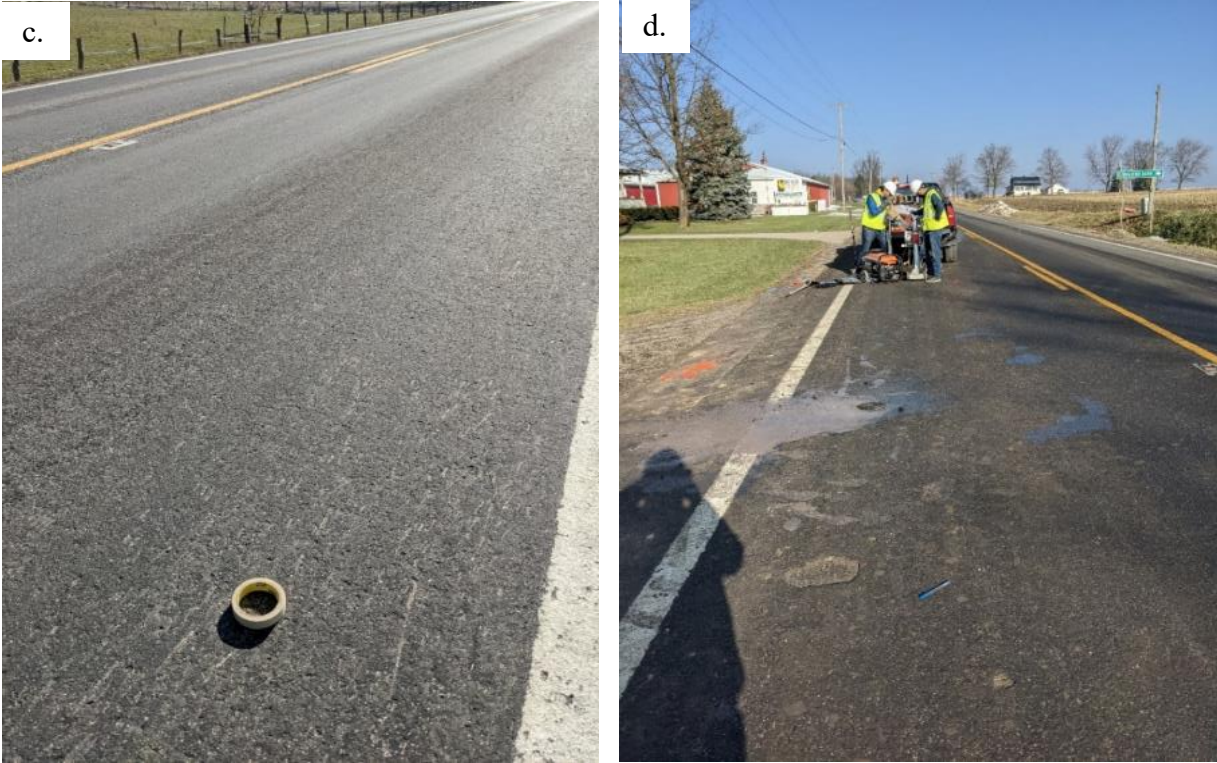
Figure B.58 photographs taken during the evaluation of deteriorated and good micro-surfacing locations at SR 89 test section and obtaining field cores from these locations: a) 16.91-16.96 SB, b) 16.6-16.61 NB, c) 15.6-16.0 SB, and d) coring at one selected location.
