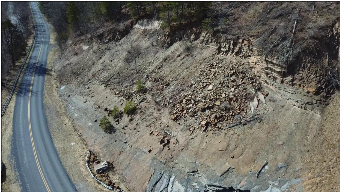
Figure 3. UAS photograph of Site #2 Route 629, Deerfield. Center right shows recent slope failure threatening anchor block for guy wires (hard to see) supporting transmission line tower out of sight.
