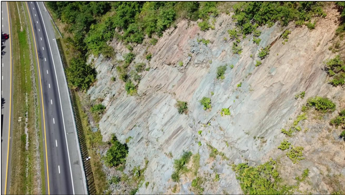
Figure 6. UAS photograph of Site #5, I-64 at MP 101 near Afton Mountain looking westbound. This is the site of previous rockslides; one of the worst occurred in 1989 and blocked the westbound lanes.
