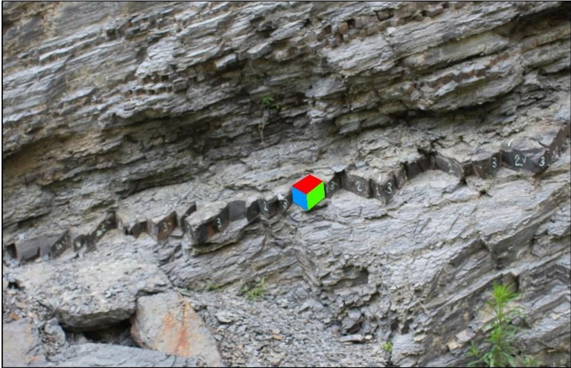
Figure 25. Site #2, Deerfield. Example of extraction of structure data from UAS-based point cloud for plotting on stereonets (Delaney, et al., 2020).
