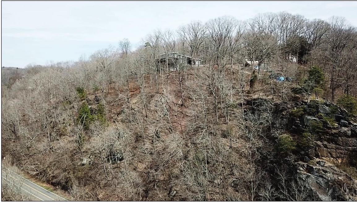
Figure 4. UAS photograph of Site #3, Route 685 River Road Lynchburg. Right side shows large rocky slope face with potential block failures controlled by the structural geology.
