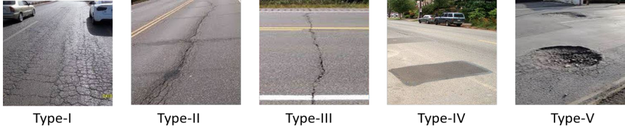
Figure 2. Pavement damage types, Type-I: Alligator Cracking, Type-II) Longitudinal Cracking, Type-III) Transverse Cracking, Type-IV) Patching, Type-IV) Potholes.
