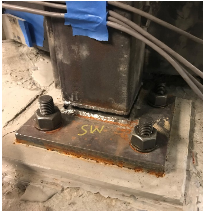
Figure 5.4: Hold-down weld failure
