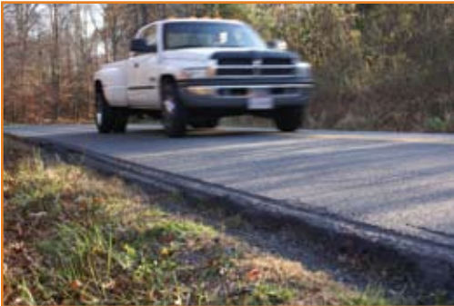
Edge drop-off on a rural road.
