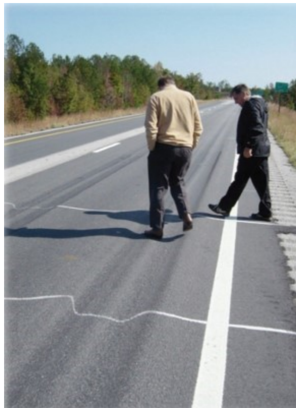
Figure 2.6. Rutting in the pavement due to high binder content and low air void in the asphalt mix (McDaniel and Levenberg 2013)
