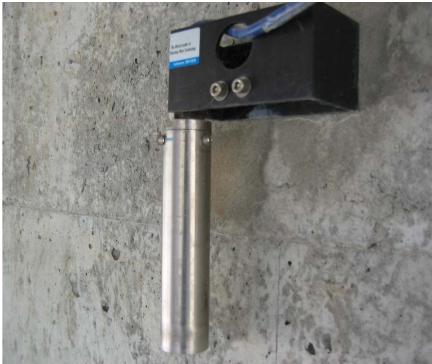
Figure 2.27: Photograph of Installed Tilt Meter and Bracket on Abutment
