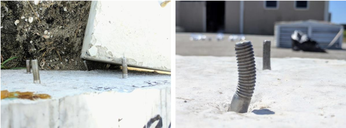
Figure 2.13 Exposure block bolts being bent (left) and bolt repaired by bending back (right)
