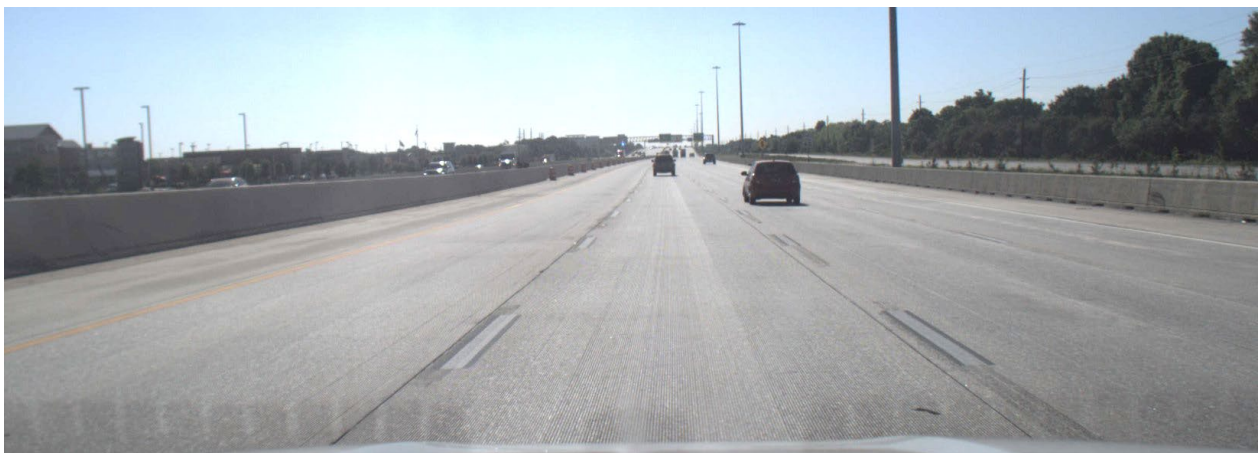
Figure 20: Image of a road segment with white pavement markings with a black border (driving eastwards).
