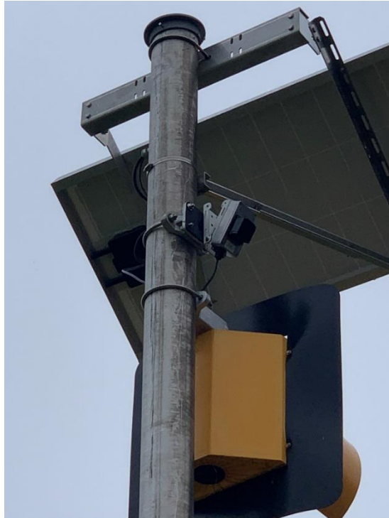
Figure 35. Example of a Sensor on the RFBA to Detect Vehicles Approaching on the Major Street.
