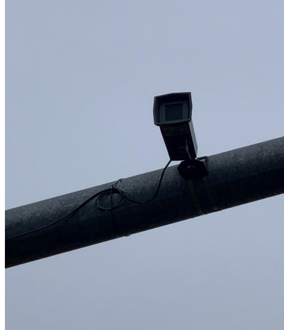
b. Sensor Installed on Mast Arm.
