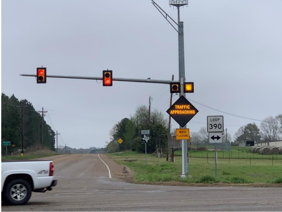
Figure 36. Example of a Warning Sign Assembly on the Minor Street (System Activated).
