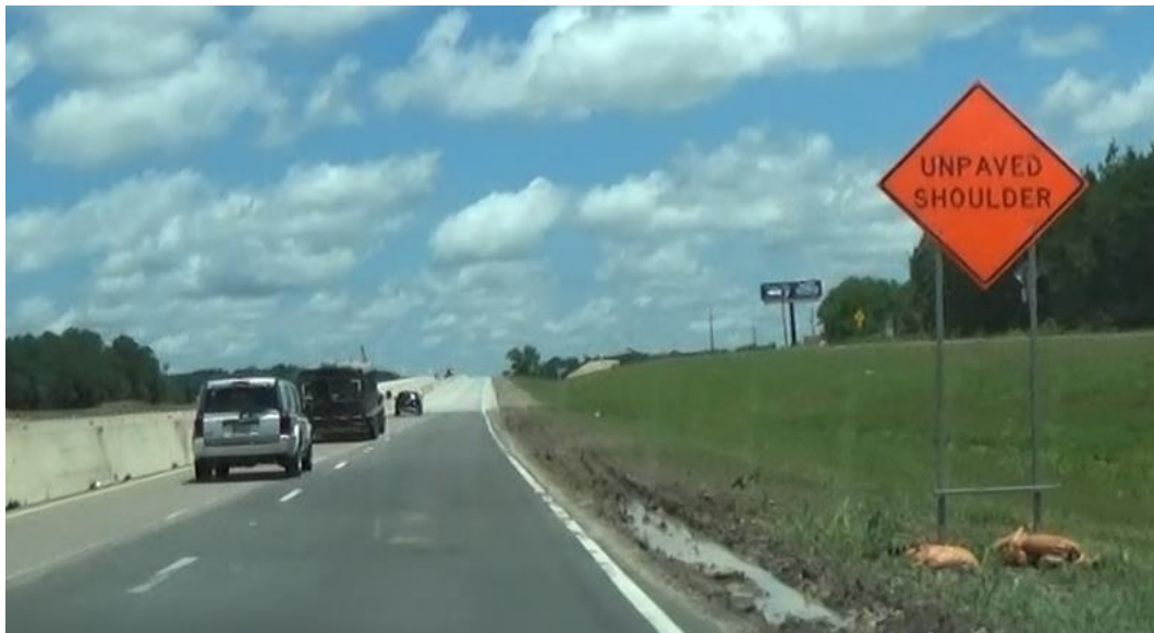
Figure 50. Unpaved Shoulder Warning Sign at Site 3.
