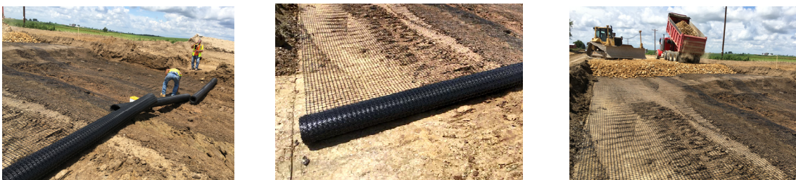
Figure 1.1: Use of geogrid in Wisconsin pavements – STH 33 between Cashton and La Crosse, WI (Pictures by Titi, 2016)
