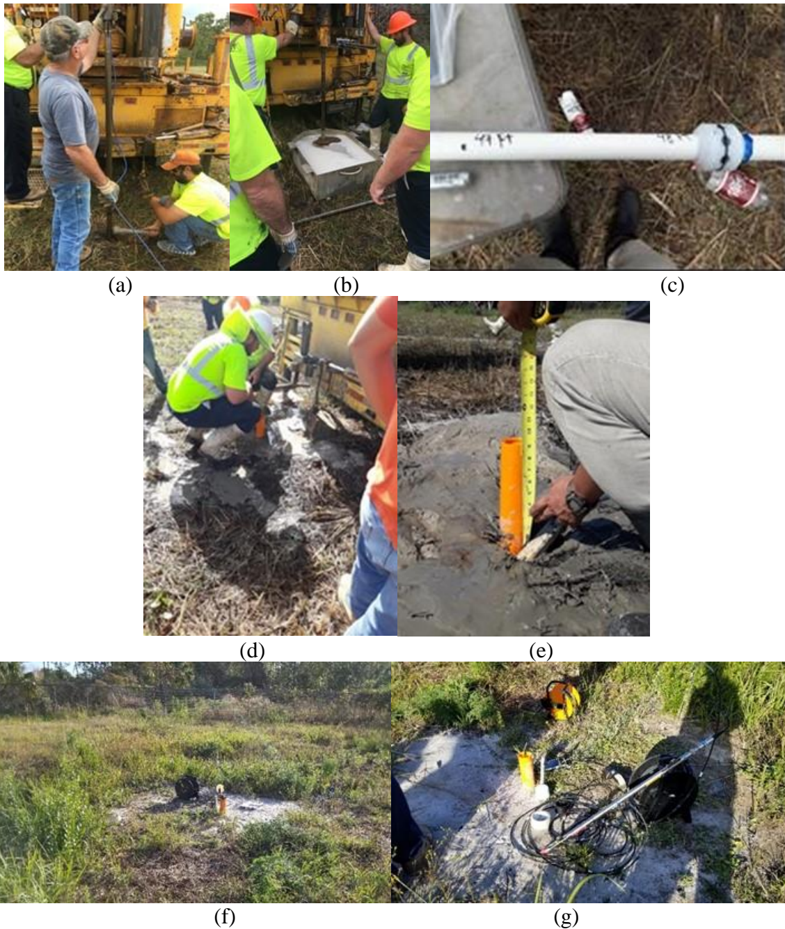
Figure 3-5. (a) Installation of piezometers in the ground using sacrificial tips, (b) drilling and grouting for installation of magnetic extensometers, (c) magnetic extensometer and datum magnet sensor, and (d-g) inclinometer casing installation
