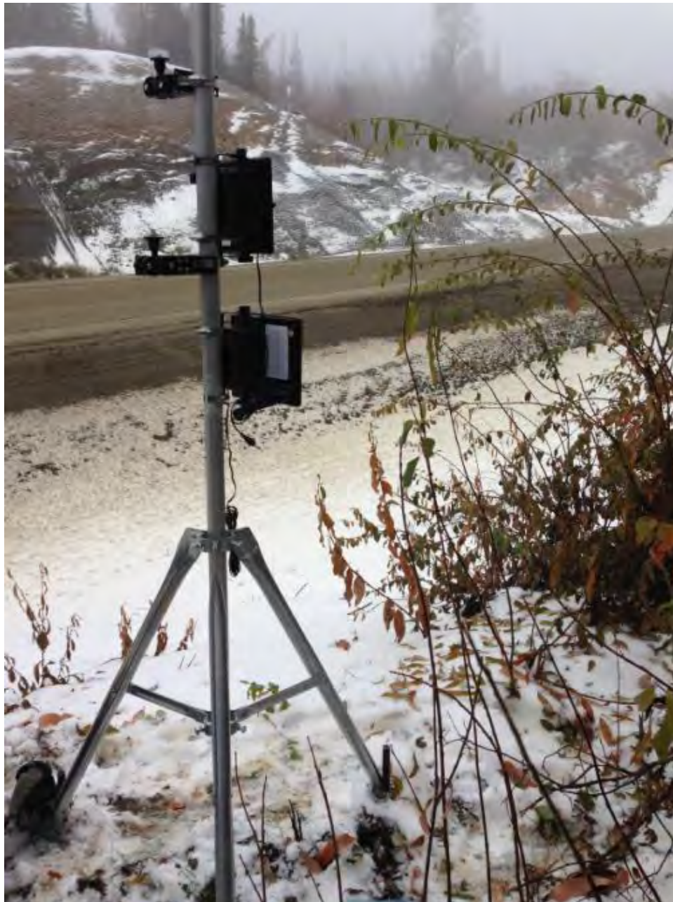
Figure 5.11 Two cameras installed for slope monitoring
