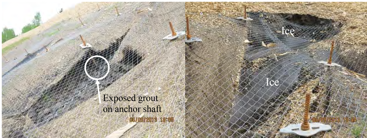
Figure 6.3 Close views showing exposure of soil anchor grout (left) and portion of massive ice feature under Tecco-mesh (right)
