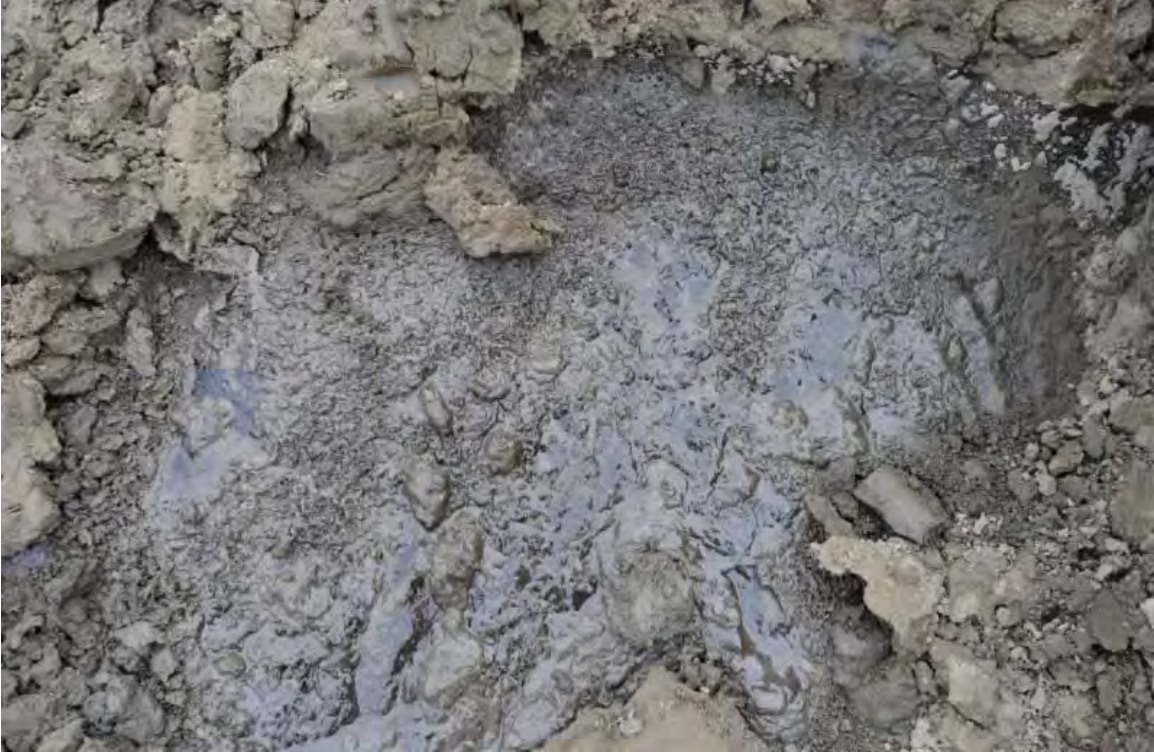
Figure 4.9 Ice exposed in the cut slope
