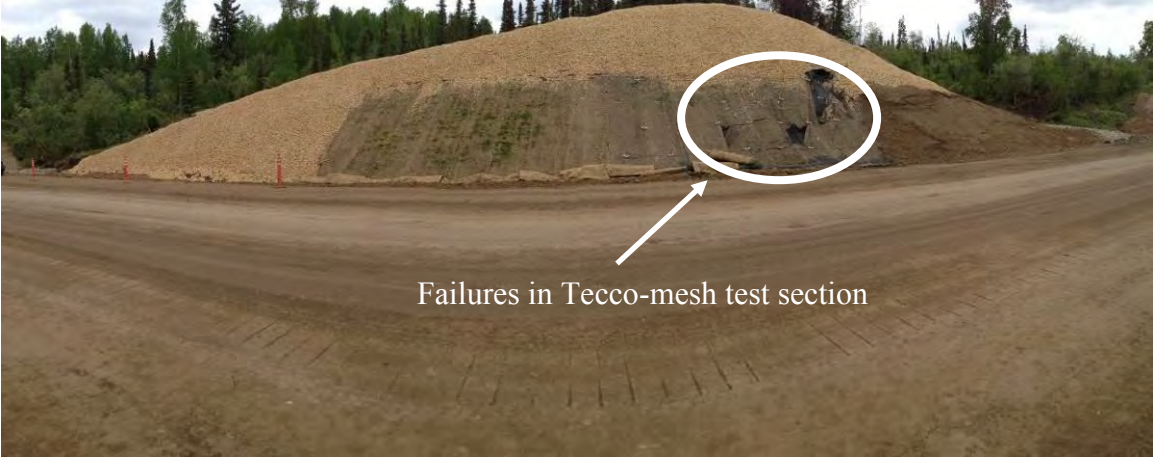
Figure 6.1 Panorama view of Experimental Feature showing failure in Tecco-mesh section
