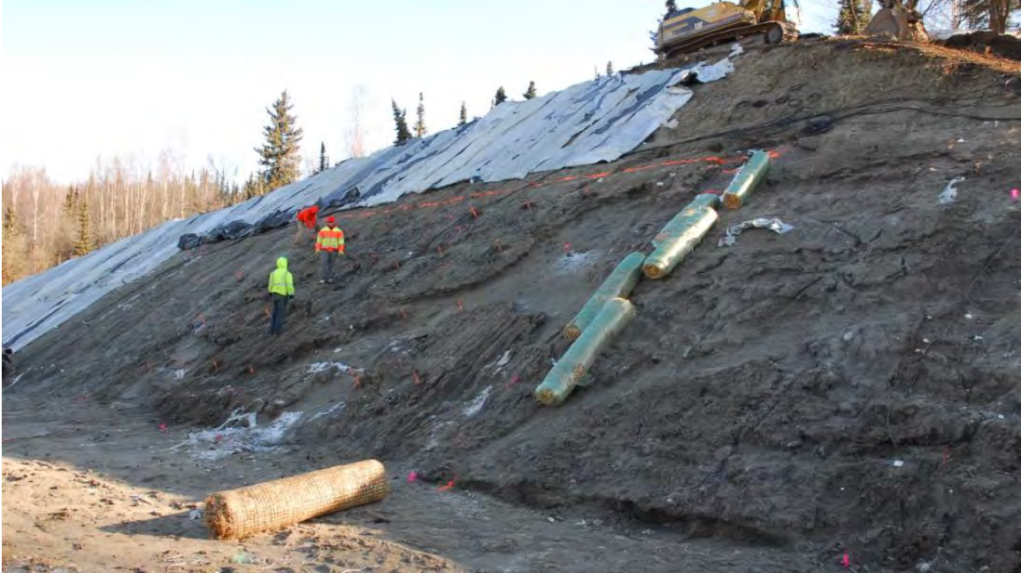
Figure 4.7 Cut slope erosion during construction
