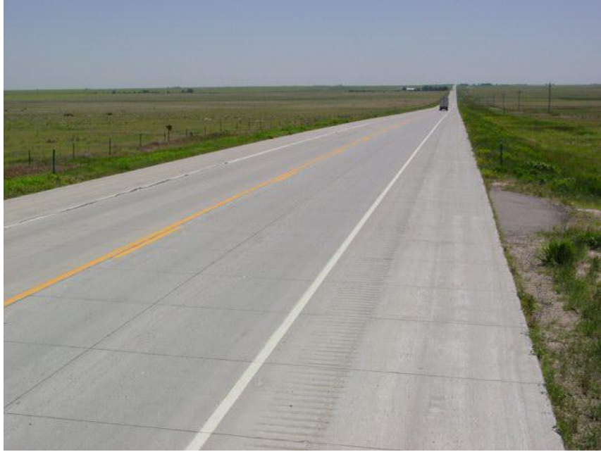
Figure 2.14 Typical Pavement Conditions Observed at the U.S. 287 Lamar Site (Sheehan et al. 2004)
