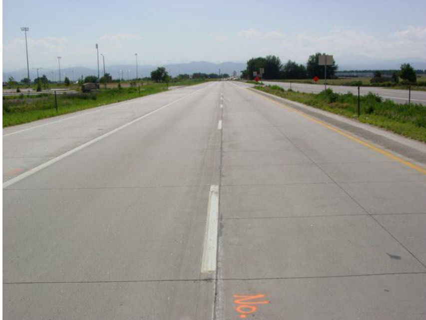
Figure 2.12 Typical Pavement Conditions Observed at the S.H. 119 Longmont Site (Sheehan et al. 2004)
