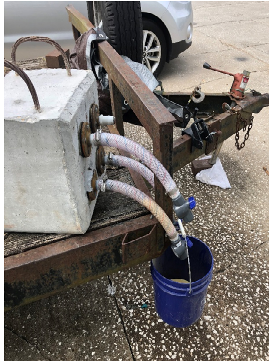
Down-stream end of tendons – photo shows two right tendons' valves closed after appearance of impregnation material. Bottom joint also shows a location of a sealed leak.
