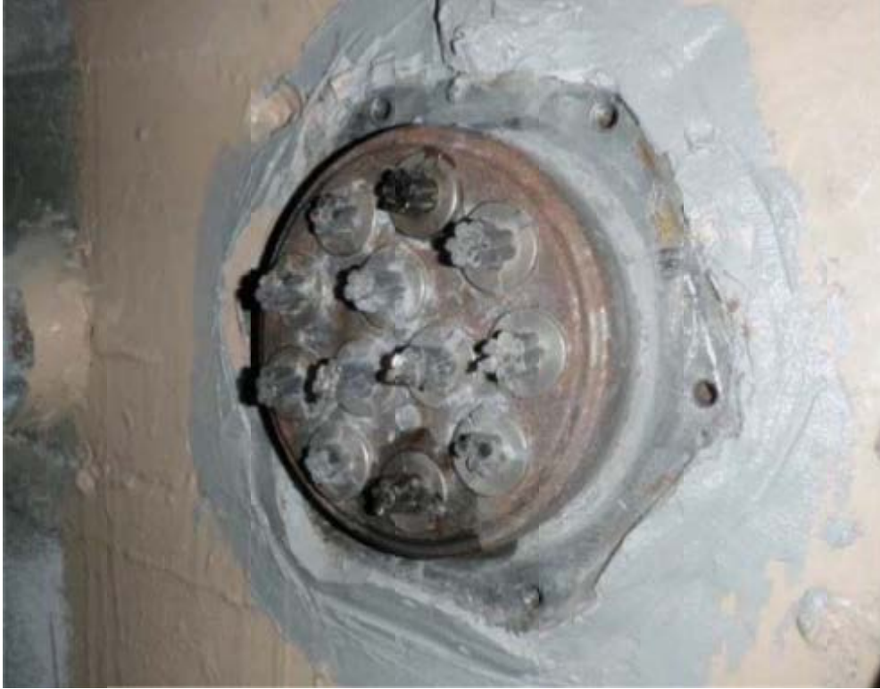
Figure 2-4: Impregnation material seep out of the far end of a >250-ft-long tendon. 47
