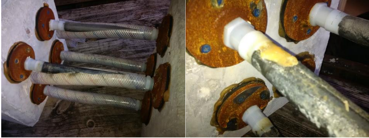
Figure 4-59: Connecting hoses removed showing residual impregnation product.
