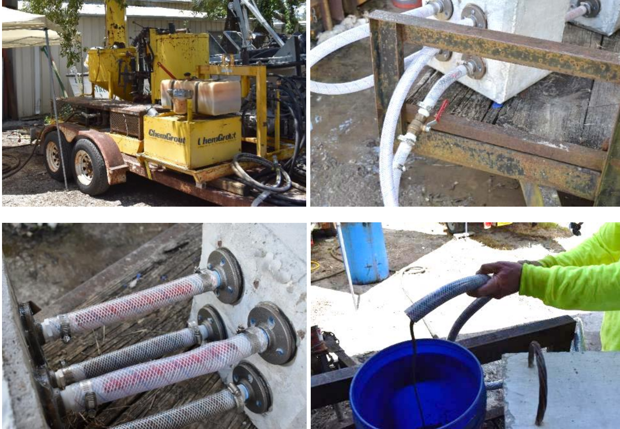
Figure 4-57: Grouting: grout plant (top left); grout hose connected to bottom duct, strand 3 (top right); grout in bottom two ducts but not yet in top two (bottom left); grout exiting four-duct system (bottom right).
