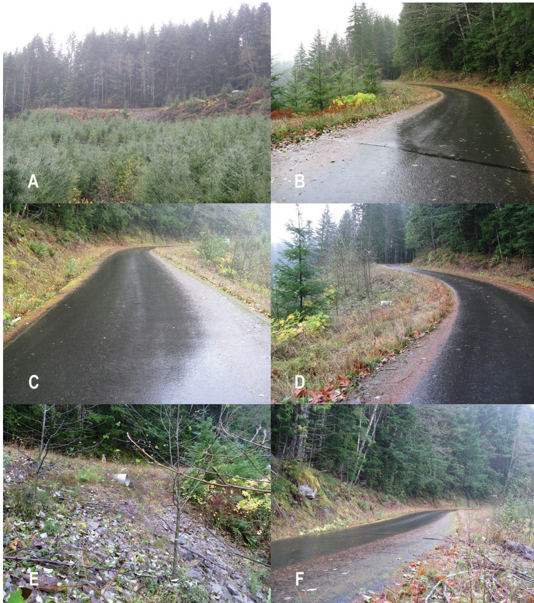
Figure 11: Photos of Road 26, Gifford Pinchot National Forest, MP 1.1 a) distant view of site from lower road, b) layout of site from end of repair, c) road surface, d) road surface with fill slope, e) fill slope showing drainage features and protective stone facing, and f) road surface with cut slope.
