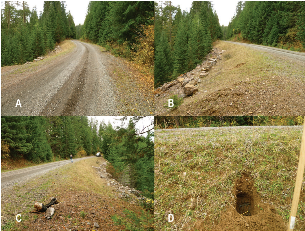
Figure 45: Photos of deep patch repairs at Site 3 on Road 6610, Rogue River-Siskiyou National Forest showing a) layout of site and road surface, b) layout of site and embankment, c) layout of site and embankment from the other end, d) geogrid reinforcement in embankment.
