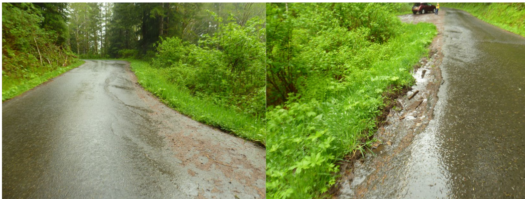
Figure 40: Photos of distresses at milepost 14.244, Road 17, Siuslaw National Forest.
