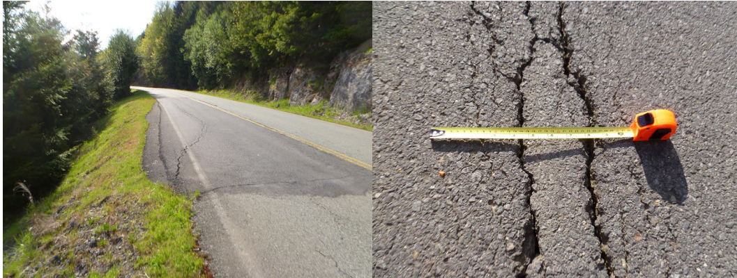
Figure 18: Photos of distresses at milepost 10.1, Road 90, Gifford Pinchot National Forest.
