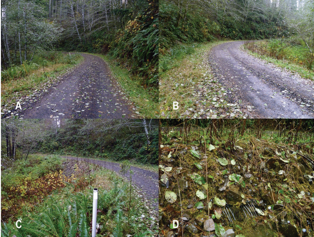
Figure 31: Photos of deep patch repairs on Road 58, Siuslaw National Forest a) layout of site from end of repair, b) layout of site looking from other end, c) fill slope showing stone facing, and d) close-up of deep patch showing exposed geogrid.
