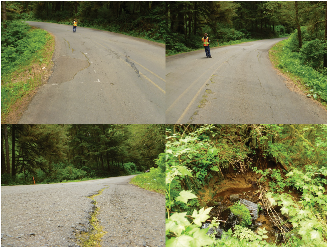
Figure 43: Photos of distresses at milepost 4.929, Road 12, Siuslaw National Forest.
