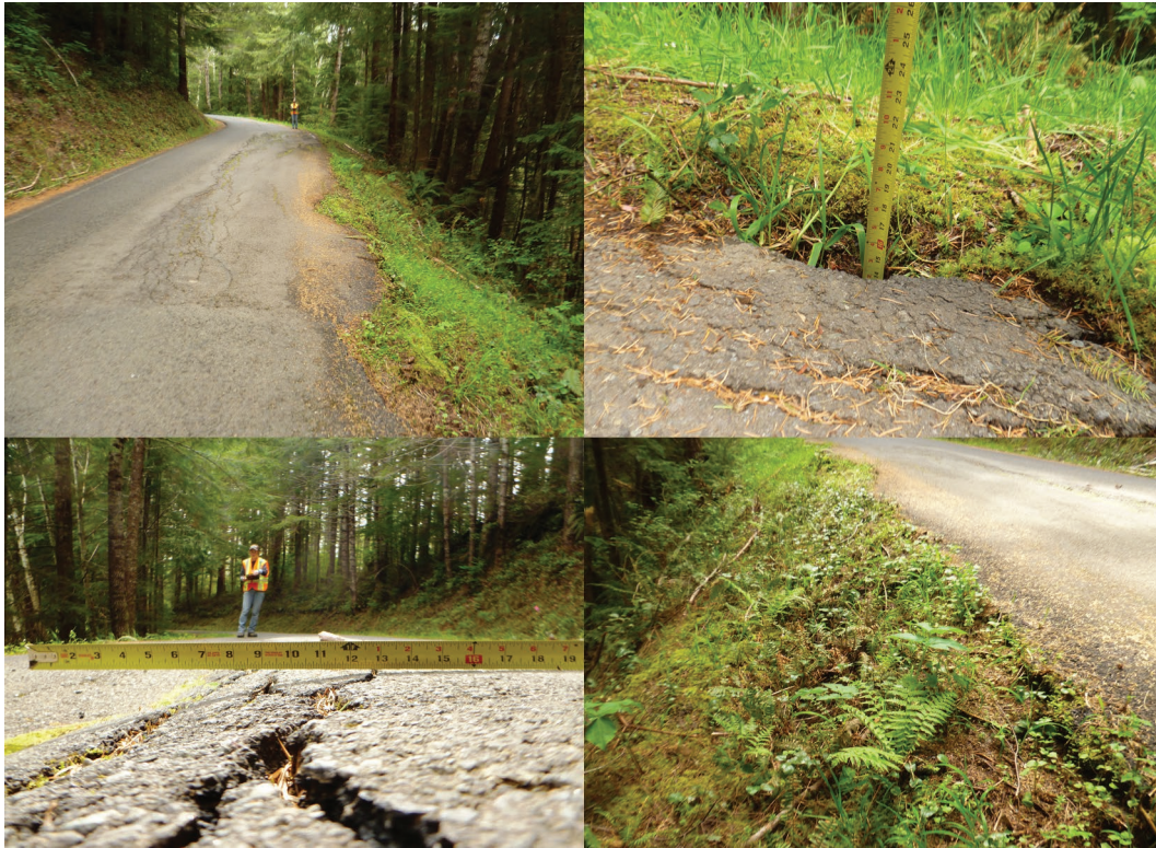
Figure 37: Photos of distresses at milepost 10.885, Road 17, Siuslaw National Forest.
