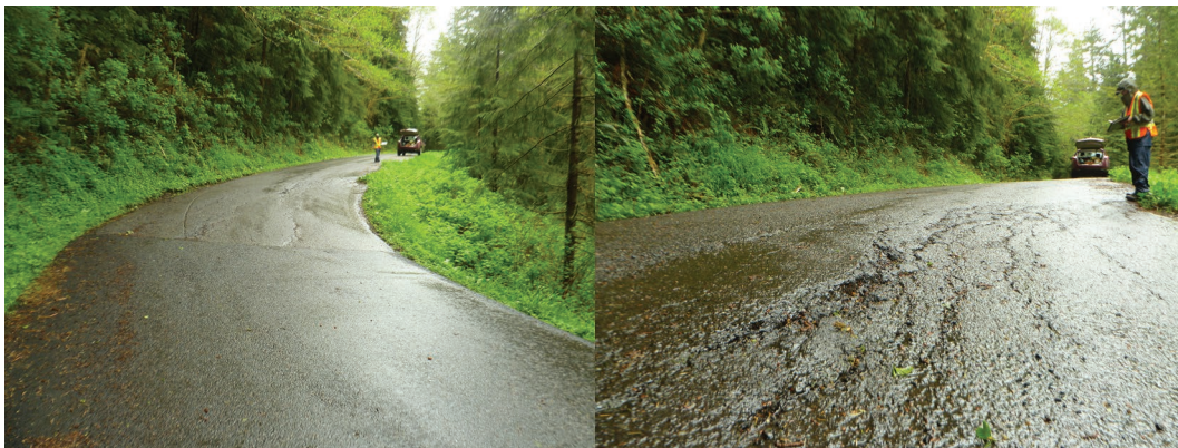
Figure 38: Photos of distresses at milepost 13.664, Road 17, Siuslaw National Forest.
