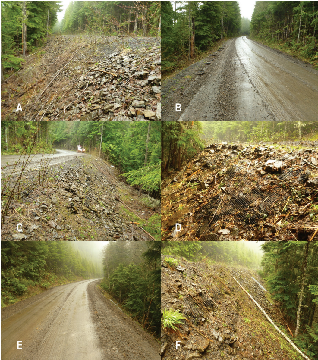
Figure 23: Photos of Road 45, Mount Hood National Forest, deep patch repairs at MP 5.85 (a, b, c) and MP 6.76 (d, e, f).
