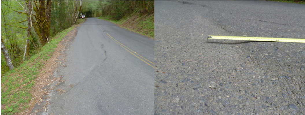
Figure 21: Photos of distresses at milepost 17.8, Road 90, Gifford Pinchot National Forest.
