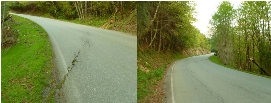
Figure 16: Photos of distresses at milepost 5.5, Road 90, Gifford Pinchot National Forest.
