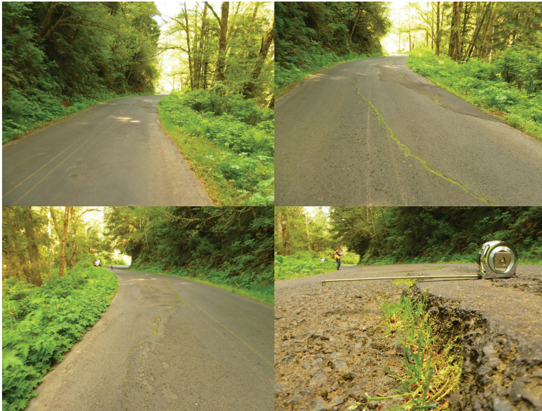
Figure 42: Photos of distresses at milepost 2.9, Road 12, Siuslaw National Forest.
