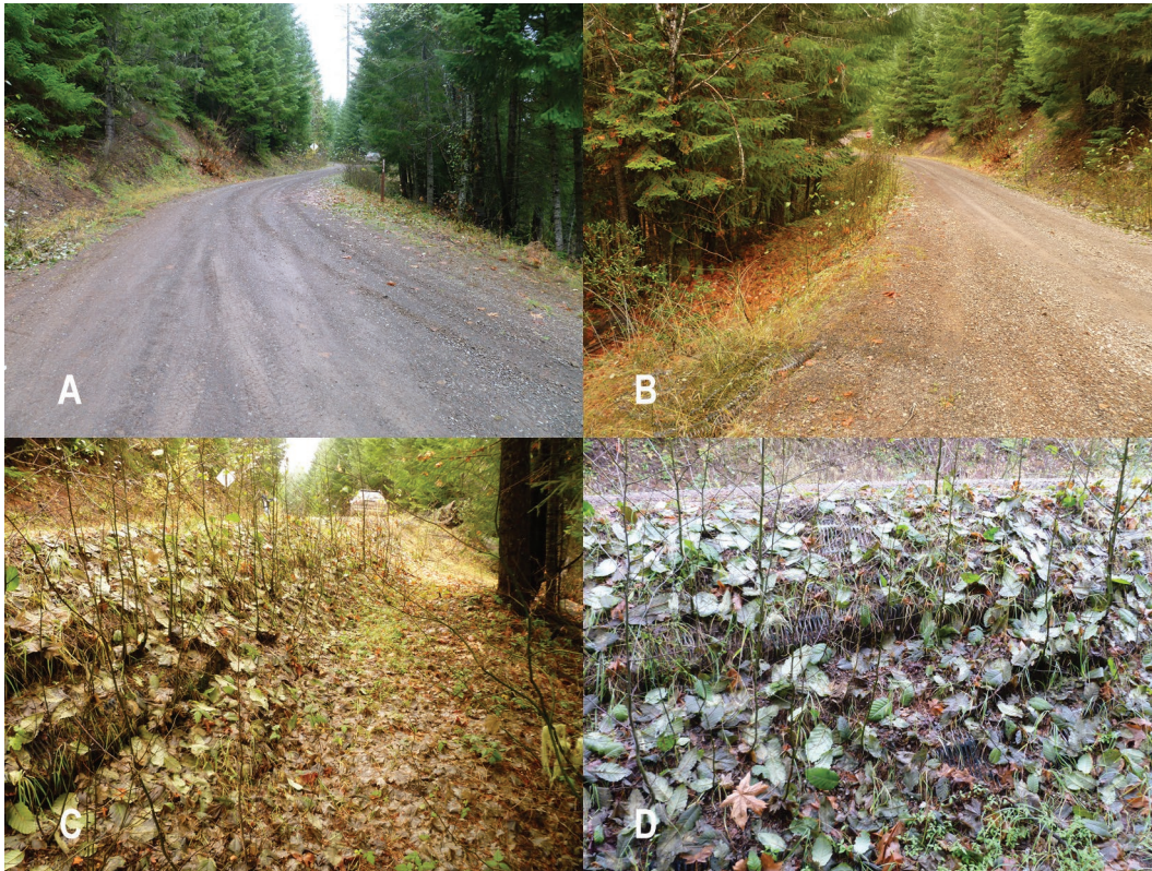
Figure 46: Photos of deep patch repairs at Site 5 on Road 6515, Rogue River-Siskiyou National Forest showing a) general layout of site and road surface, b) layout of site from other direction (note geogrid in foreground that was unearthed by grader), c) embankment, d) exposed geogrid reinforcement in embankment.
