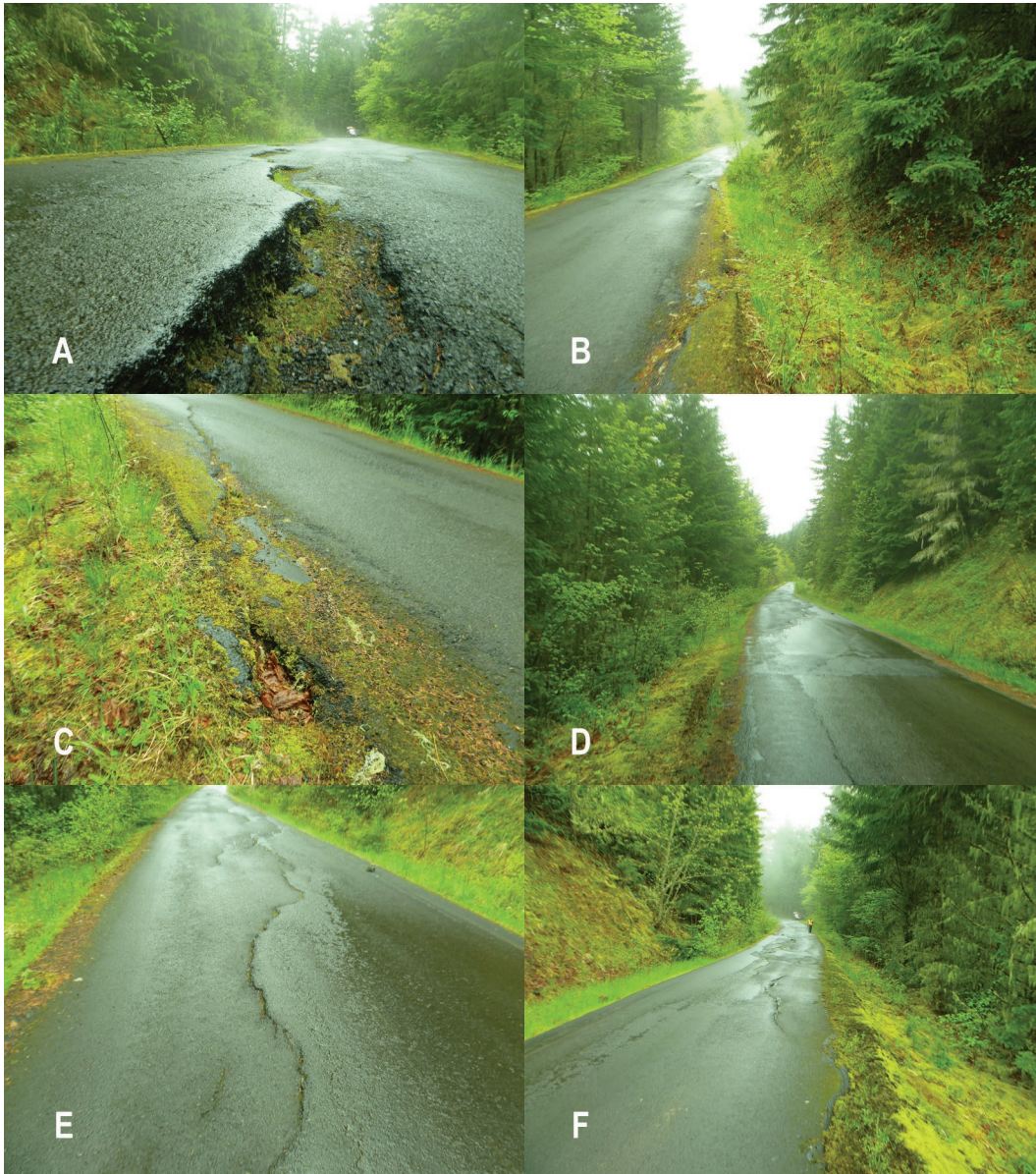
Figure 26: Photos of distresses on Road 45, Mount Hood National Forest, MP 28.2 a) close-up of differential settlement at crack interface, b) crack extending to inside shoulder, c) close-up of crack at inside shoulder, d) general view of road surface distresses, e) surface cracking and f) general view of surface distresses.
