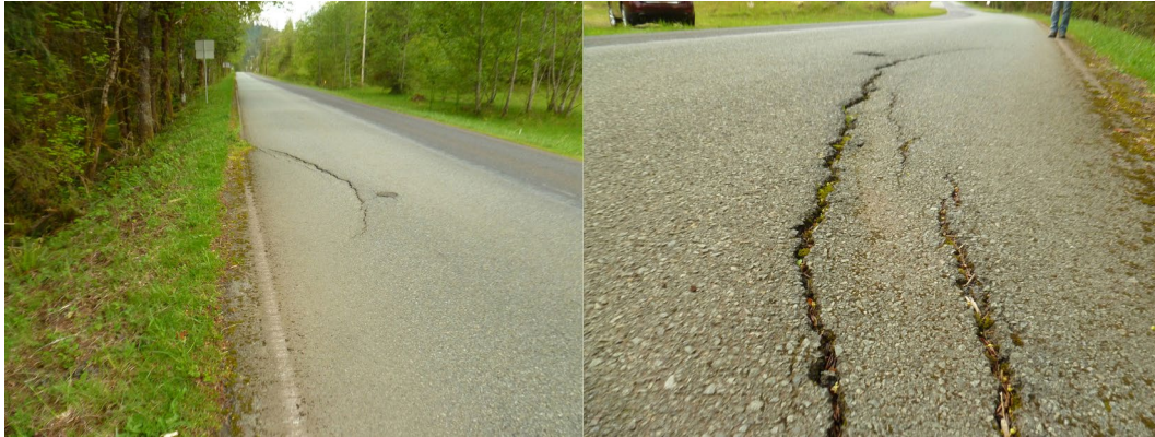
Figure 15: Photos of distresses at milepost 0.1, Road 90, Gifford Pinchot National Forest.
