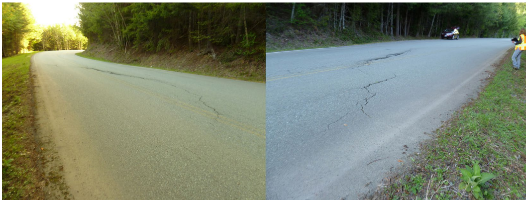
Figure 17: Photos of distresses at milepost 6.3, Road 90, Gifford Pinchot National Forest.
