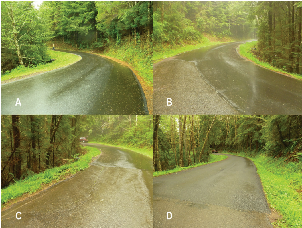
Figure 34: Selected photos of repaired sites on Road 17, Siuslaw National Forest: a) MP 9.14, b) MP 9.39, c) adjacent distresses near repair at MP 9.39, d) MP 9.65.
