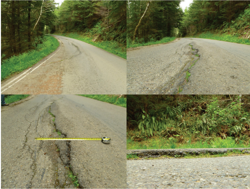
Figure 41: Photos of distresses at milepost 14.413, Road 17, Siuslaw National Forest.
