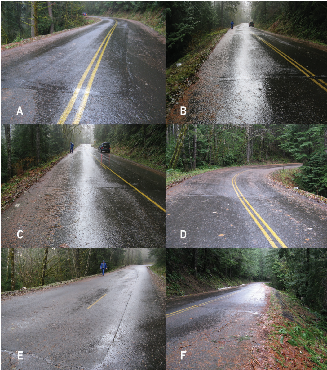
Figure 14: Photos of Road 25, Gifford Pinchot National Forest deep patch repairs at a) MP 9.158, b) MP 9.228, c) MP 9.252, d) MP 10.032, e) MP 10.898, and f) MP 11.509.
