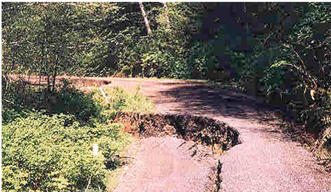
Figure 28: Photo of slope failures on Road 58, MP 29.65, Siuslaw National Forest.
