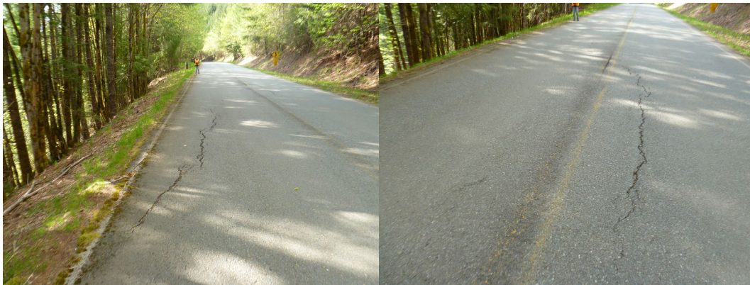
Figure 19: Photos of distresses at milepost 11.9, Road 90, Gifford Pinchot National Forest.
