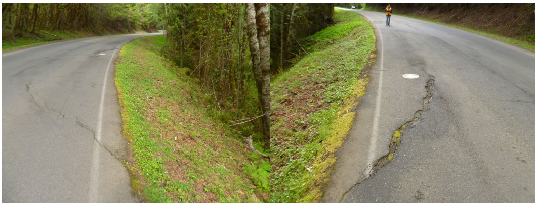
Figure 20: Photos of distresses at milepost 14.1, Road 90, Gifford Pinchot National Forest.
