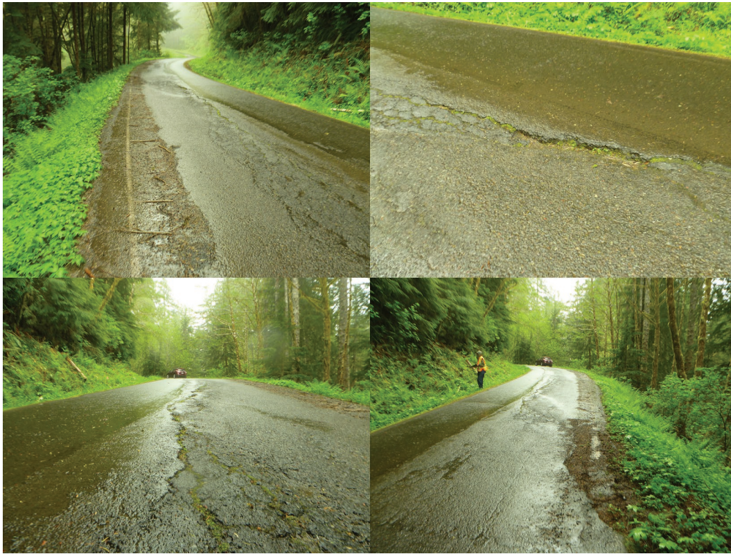
Figure 39: Photos of distresses at milepost 13.851, Road 17, Siuslaw National Forest.
