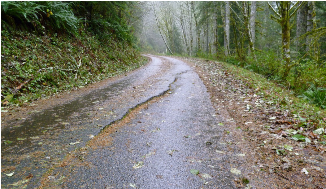
Figure 3: Common fill slope distress on sidecast constructed road.
