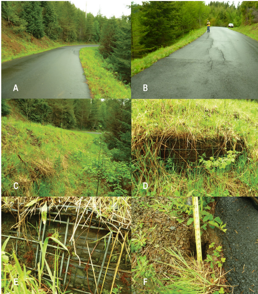
Figure 35: Photos of deep patch repairs at milepost 7.92 on Road 17, Siuslaw National Forest showing a) layout of site from end of repair, b) layout of site looking from other end, c) fill slope showing vertical facing, d) welded wire mesh to provide vertical support of slope face, e) close-up of vertical wire mesh showing geosynthetic reinforcement and separation geotextile, and f) hole near outside edge of pavement.
