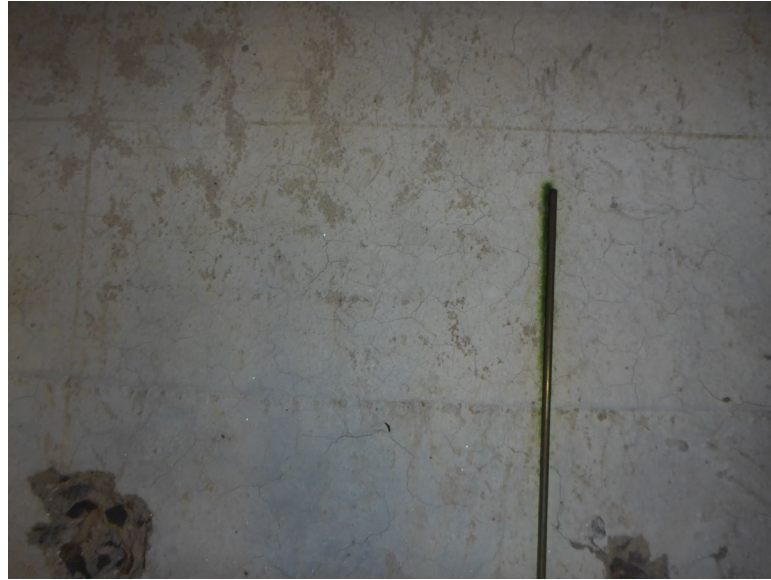
Figure 7.14: Typical map cracking pattern for slabs after heating up to 930°C
