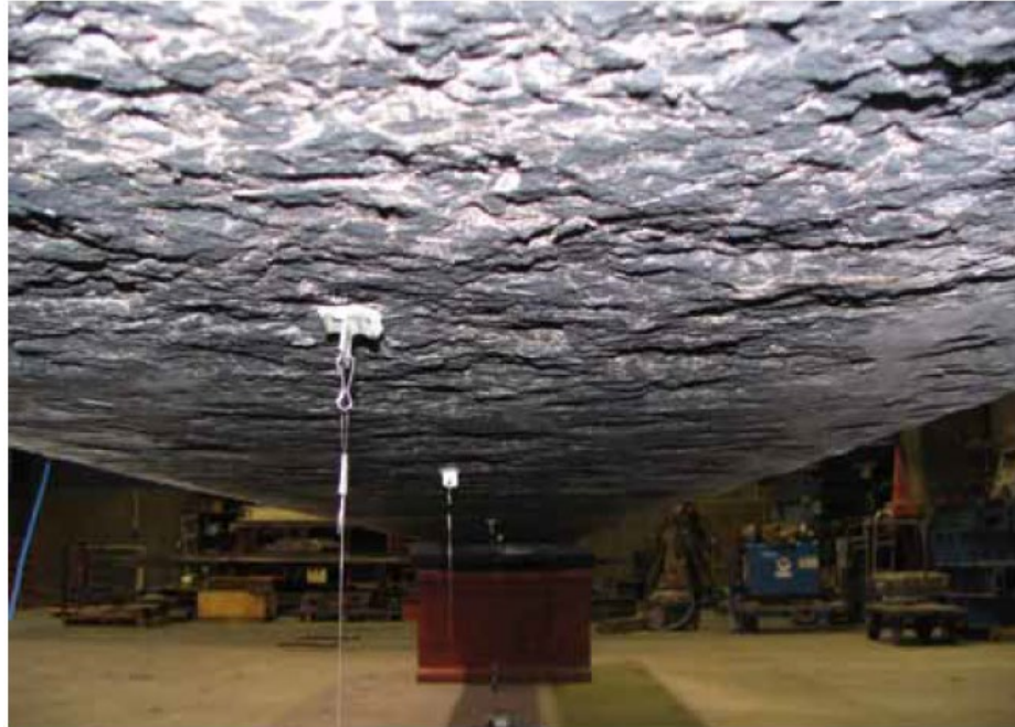
Figure 3.9: Visual condition of bottom of Beam 4, Ridgefield bridge
