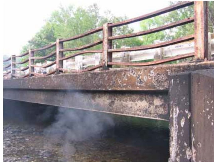
Figure 3.7: Fascia of Ridgefield, CT, bridge after the fire
