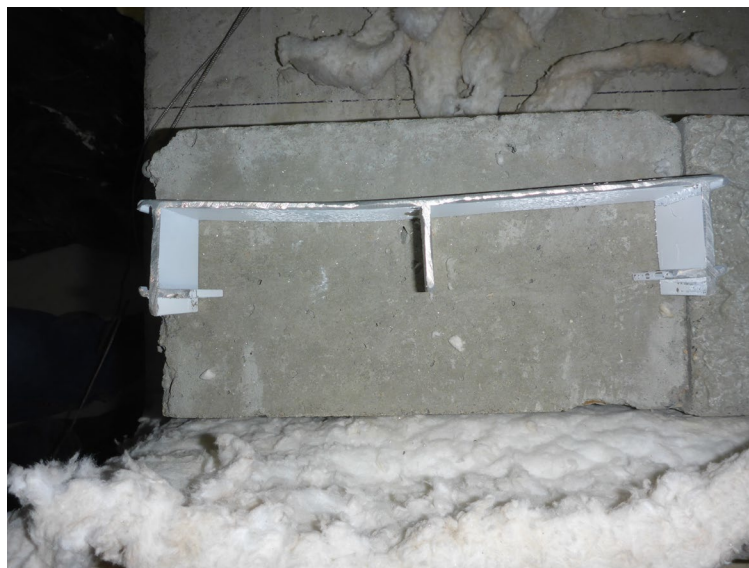
Figure 7.20: Sagging of aluminum wireway after heating
