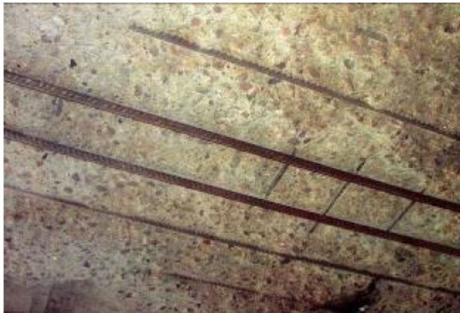
Figure 5.1: Buckled reinforcing bars in underside of slab
