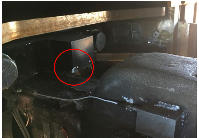
Figure 15. Damage to the limit stop mounted to the front of the sliding lug due to contact by the back of the PBC coupler head
