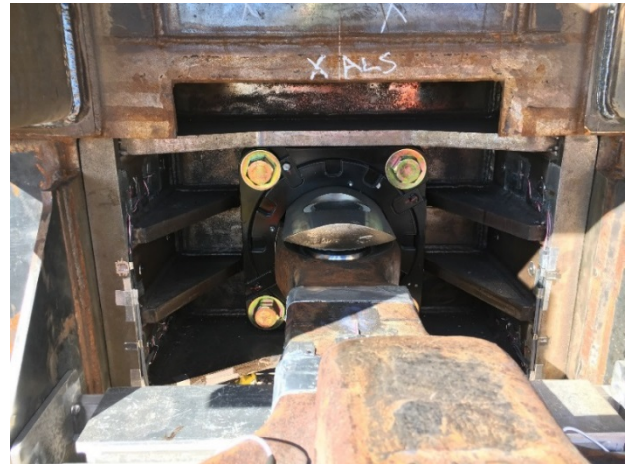
Figure 7. PBC installed within the sliding lug
