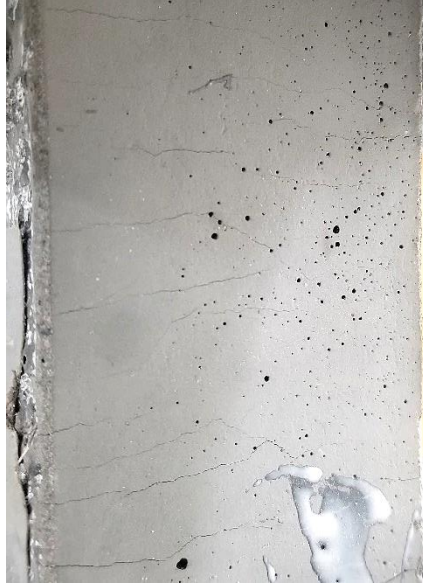
Figure 2-11 Multi-cracking during uniaxial tensile loading (Photo credit: Torres)
