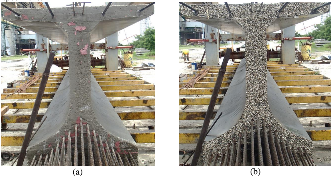
Figure 4-7 SCC surface preparation: (a) Prior to water jetting and (b) After water jetting
