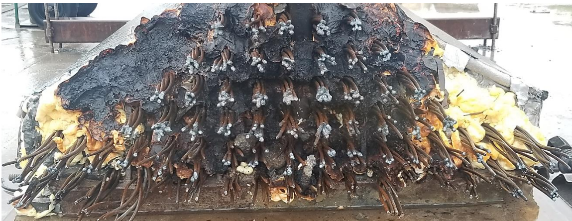
Figure 3-21 Photo of prestressing strands after strand rupture
