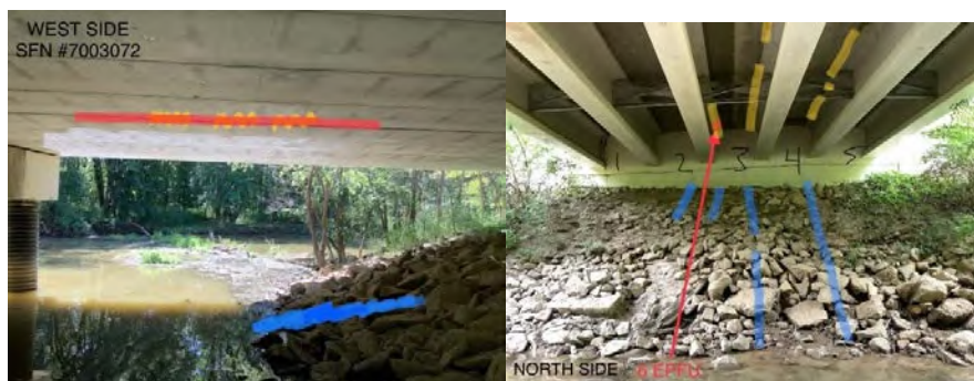
Typical images of ODOT bridges used by bats. A box beam bridge is shown on the left; the right is an I-beam bridge; both cross streams and abundant habitat exists within the immediate area. NOTE: the added colors show places where bats (red), staining (yellow), and guano (blue) were observed.
