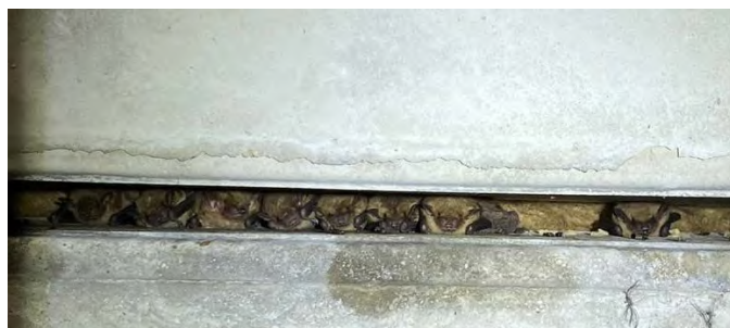
Big brown bats in a Box Beam Bridge. Note staining on concrete and insulation.
