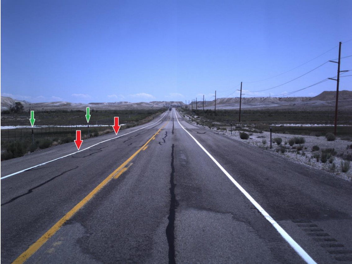
Figure 4.13 Photograph looking northbound (positive direction) of patch area with IRI undulation in the negative direction of travel indicated by red arrows. Culvert markers are indicated by green arrows. (Courtesy of UDOT/Mandli Communications)
