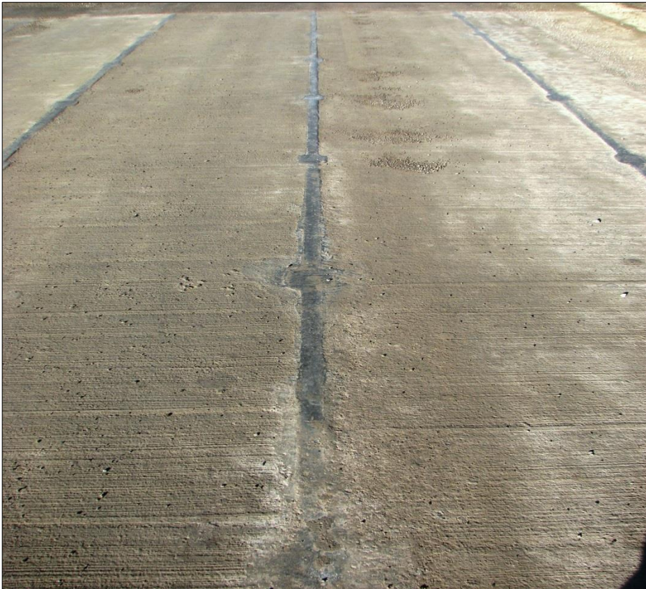
← Once all ties were welded the gap in the slab joints were plugged with foam backer rod then filled with non-shrink grout as seen in this image.
