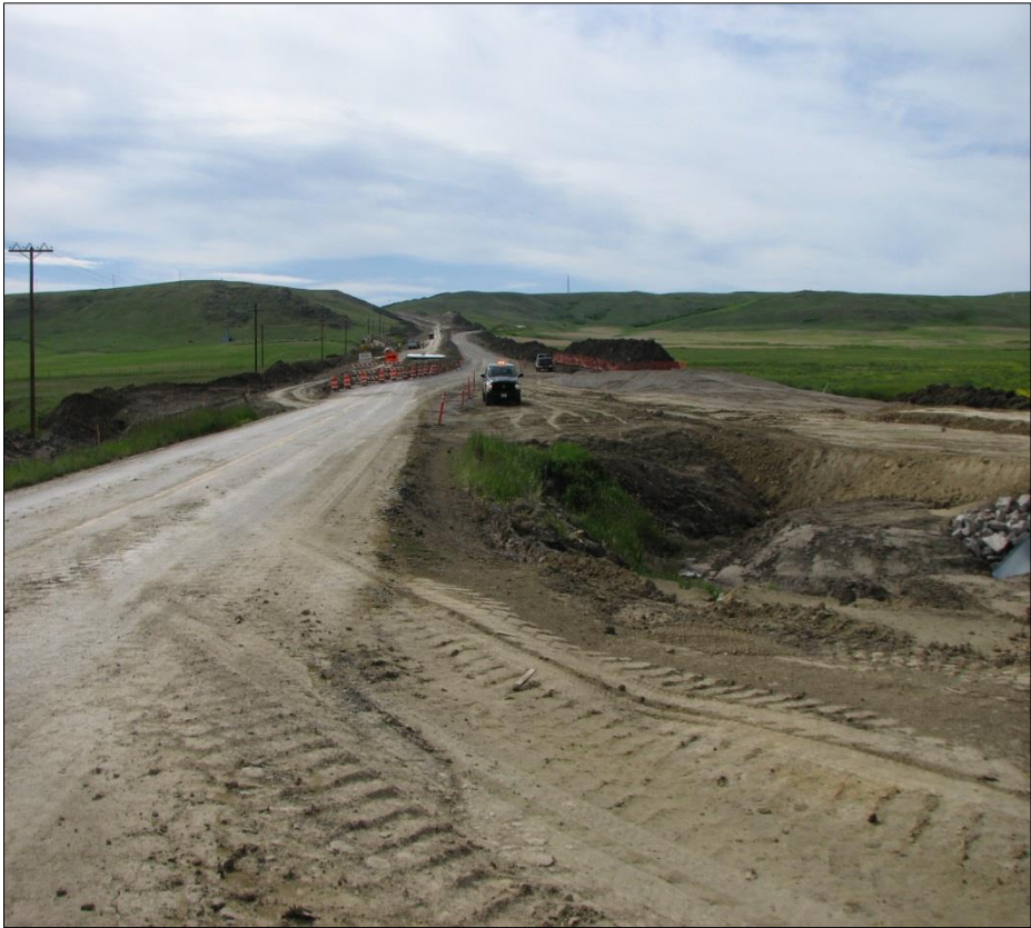
← A temporary detour directly adjacent (west) to the GRS bridge site is put in place.
