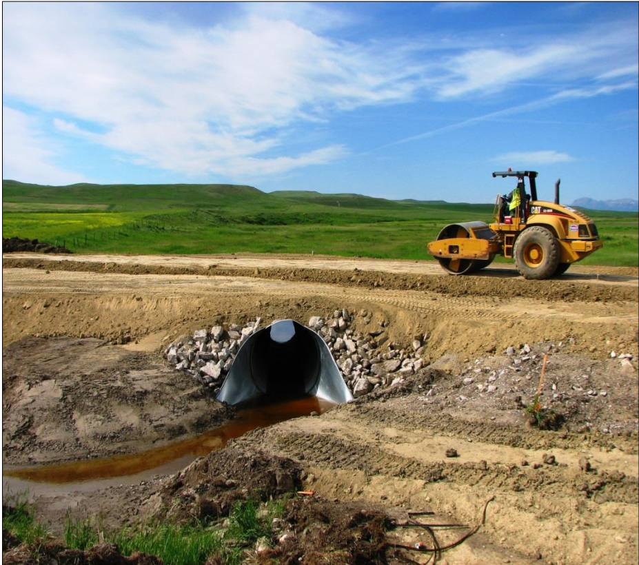
← A culvert was installed in the detour to transfer the stream which normally is dry but did have standing water at the time of this documentation. Rip rap was added, and later straw wattles were included.
