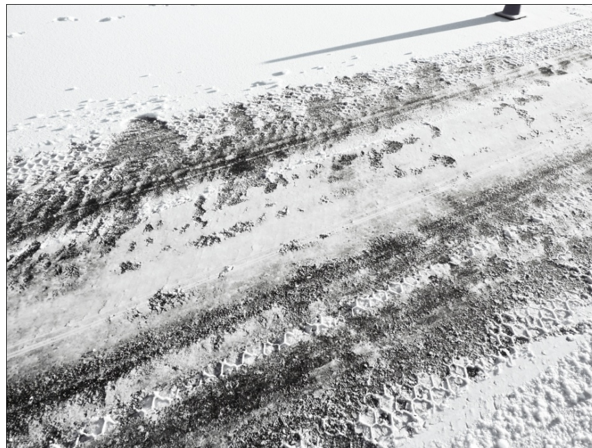
Figure 44: Snow remaining on test section due to uneven asphalt surface.
