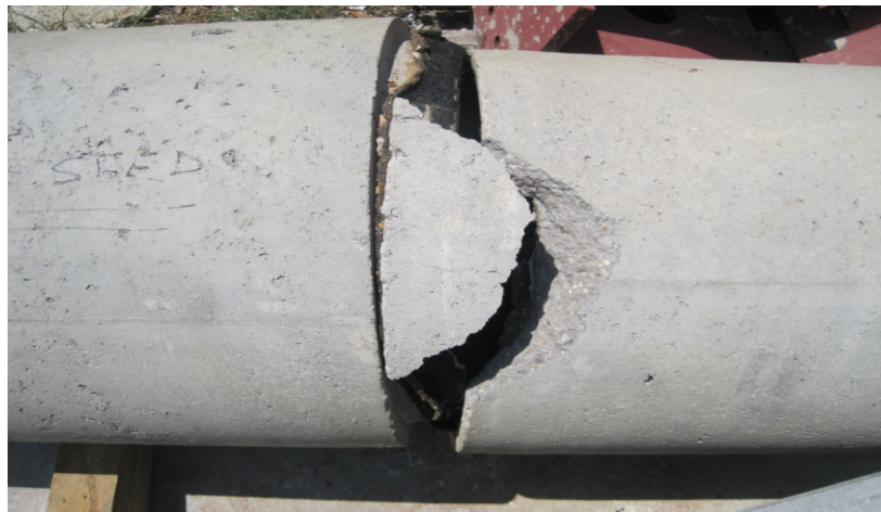
Figure 57. Concrete Pipe Fatigue Damage Observed.
