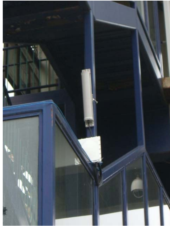
Figure 19: Proxim Pre-WiMAX base station antenna installation - Close-up view
