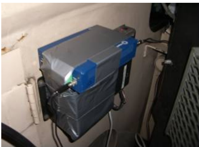
Figure 25: IndigoVision Video Encoder installation in Locomotive V02
