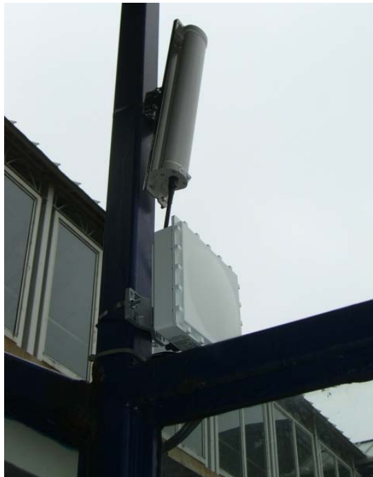
Figure 20: Proxim Pre-WiMAX base station antenna installation - Side view
