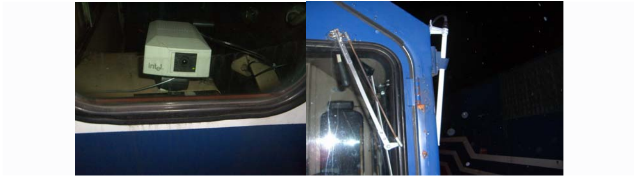
Figure 5: Camera and Antenna - Locomotive
