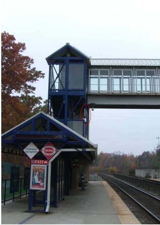
Figure 18: Proxim Pre-WiMAX base station and antenna installed at Franconia-Springfield Station
