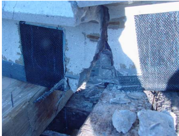
FIGURE 5.8. CFRP rupture of Beam 2.
