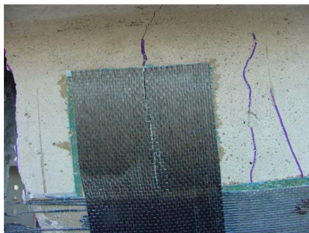
FIGURE 5.37. Flexural cracks held together by stirrups at failure
