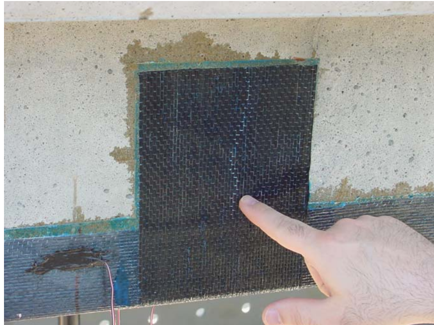
FIGURE 5.29. Existence of concrete flexural cracks in the constant moment region behind the external stirrups that developed during cycling.
