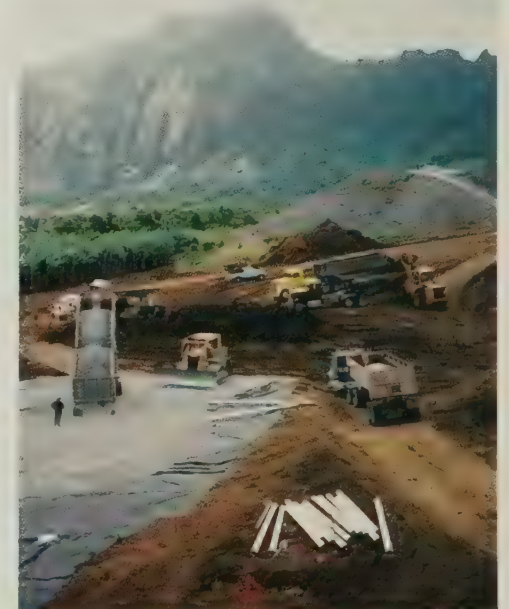
Construction on the Kaneohe interchange which is one of 20 contracts for the H-3 project. The shear windward side of the Koolau Mountains is in the background.
