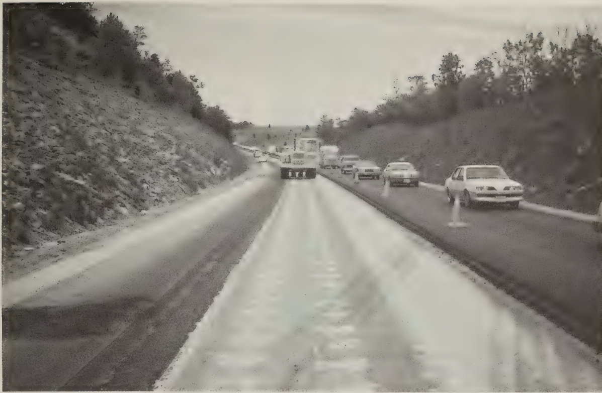
Substantial resurfacing and rehabilitation programs will be required to maintain pavement structure in an acceptable condition.
