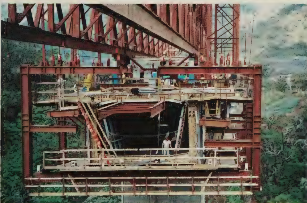
Top. A view of the steel cantilevered truss used to construct the North Halawa Valley Viaducts.
