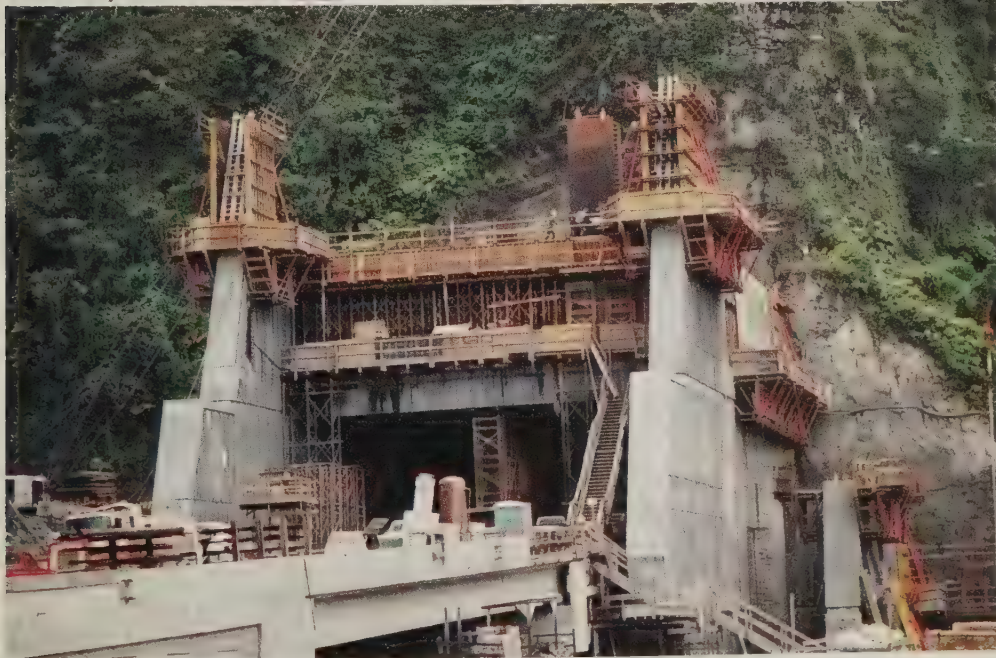
Top. The twin Windward Viaducts looking away from the tunnels. Center. The portal buildings on the windward side. Bottom. The outbound, windward side portal structure.
