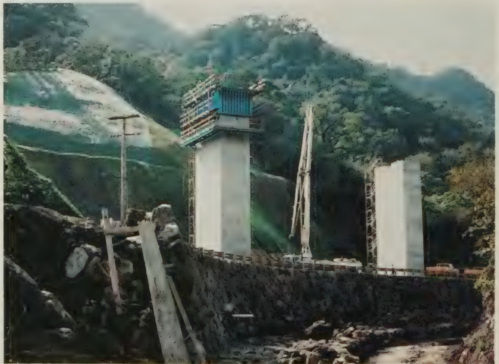
Construction of the North Halawa Valley Viaducts piers and stream bank protection.
