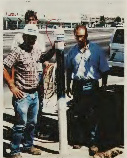
A fiber-optic sensor being emplaced at a busy intersection in Albuquerque.
