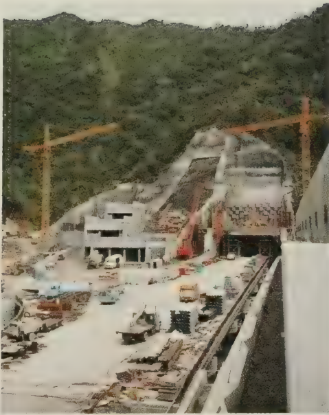
The control building and outbound portal on the North Halawa or leeward side of the Trans-Koolau Tunnels.
