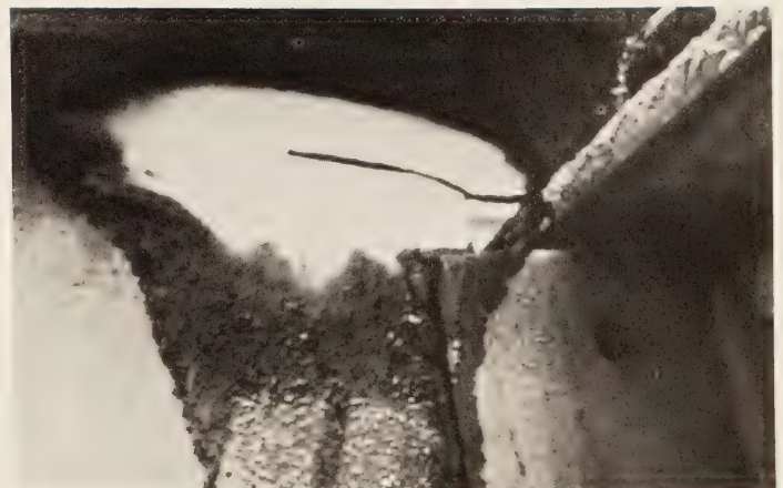
Figure 4.—Use of dye penetrant revealing the extent of a crack in a coped web.
