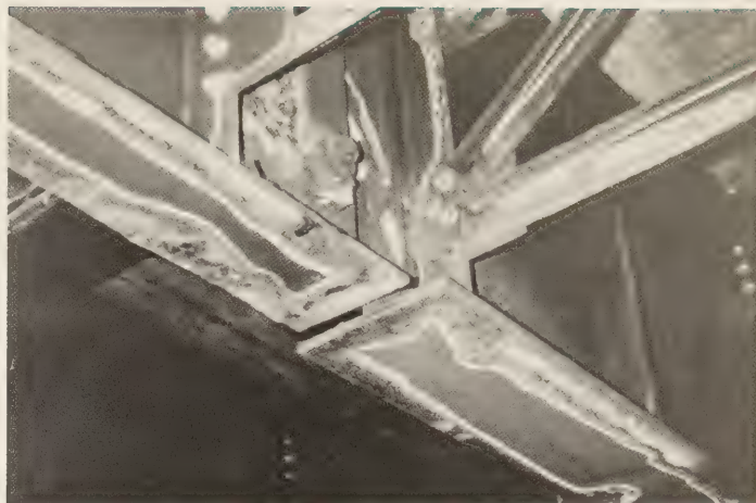
Figure 1.—A leaking expansion joint allowed road salts to deposit on these steel bridge members.
