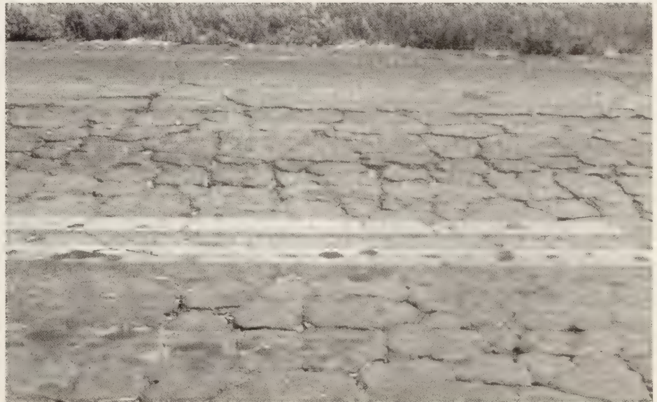
Pavement sections with high alligator cracking.
