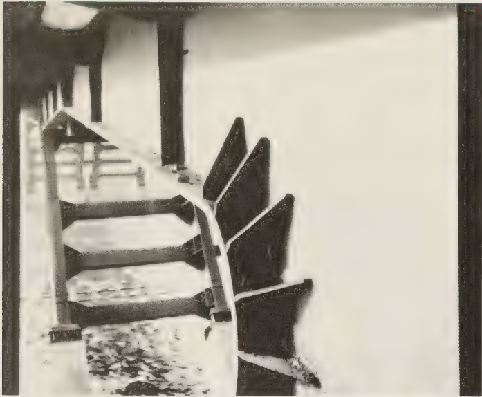
Figure 4.—These stiffeners can trap water.
