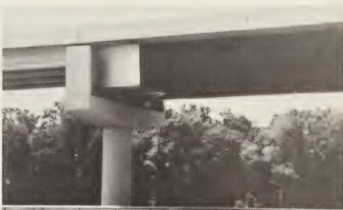
Figure 2.—Weathering steel members painted near an expansion joint.
