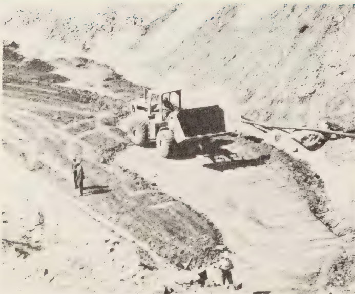
Figure 5. — Construction of the first Reinforced Earth wall in the United States (along State Highway 39 in California).
