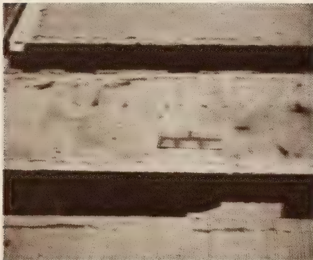
Figure 14.—Slab 234: Black steel, both mats, 11.3 kg CF/m 3 (19 lb CF/yd 3 ), April 1982.
