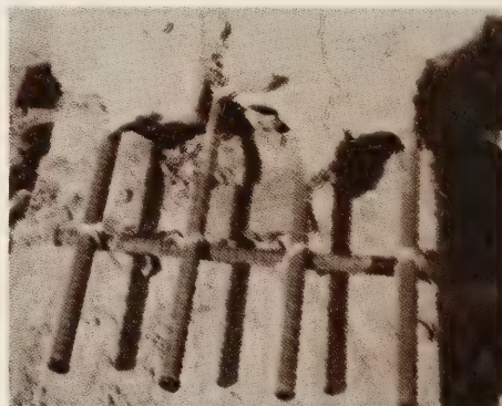
Figure 11.—Slab 204: Demolished, no visible rust on epoxy-coated rebars.
