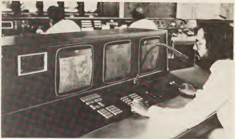
Figure 2.—ANF operating and control desk at EMS communications center.
