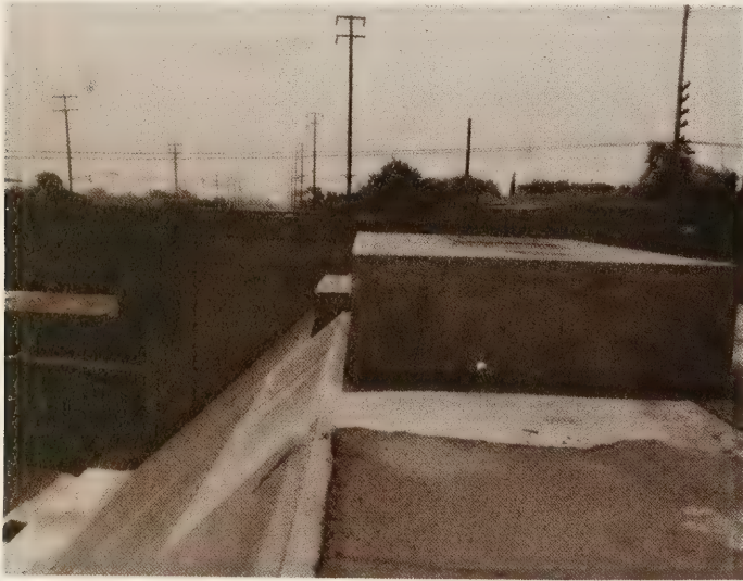
Figure 10.—Wet-pit station retrofitted to dry-pit.
