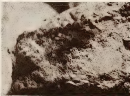
Figure 9.—Slab 201: Demolished, concrete with rebar rust imprint.
