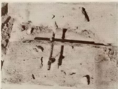
Figure 8.—Slab 201: Demolished, visible rust on iron rebar mat.
