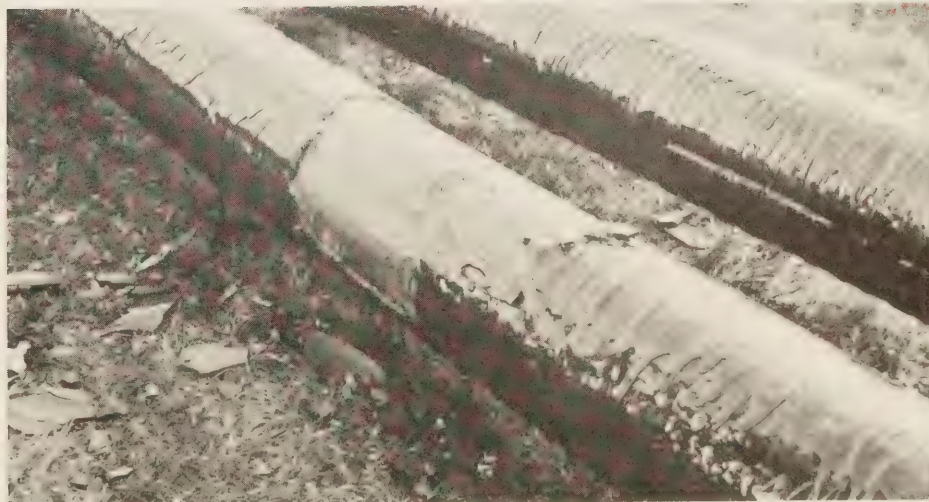
Figure 5.—Effects of using "brittle" bitumen without primer. Lack of adhesion evident.
