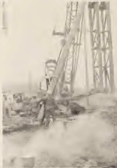
Figure 7.—Lower section of test pile No. 2 being lifted into leads. Hot bitumen ready for repair of coating.
