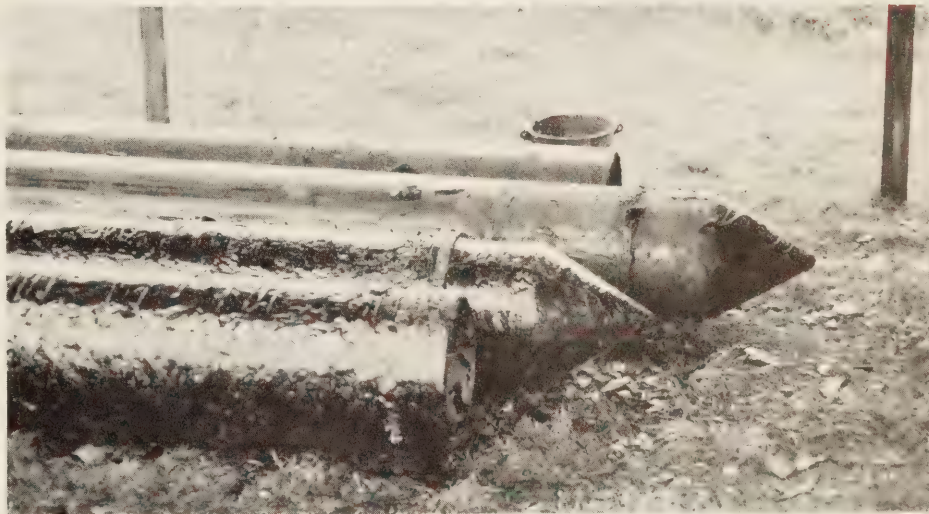
Figure 4.—Unsatisfactory coating from using "brittle" bitumen and no primer.
