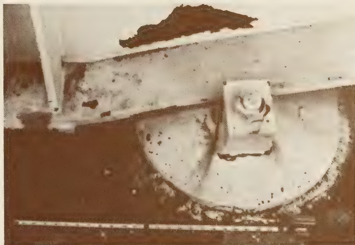
Figure 10.—Longitudinally displaced girder.
