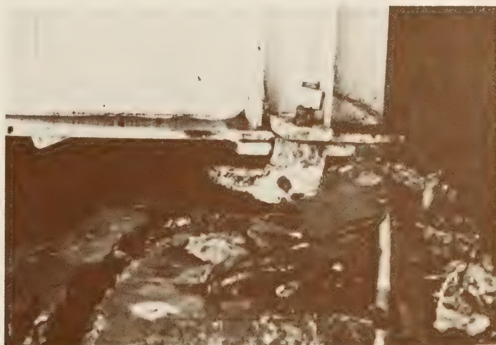
Figure 11.—Abutment movement and damage.
