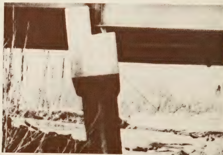
Figure 1.—Pier or column tilting.
