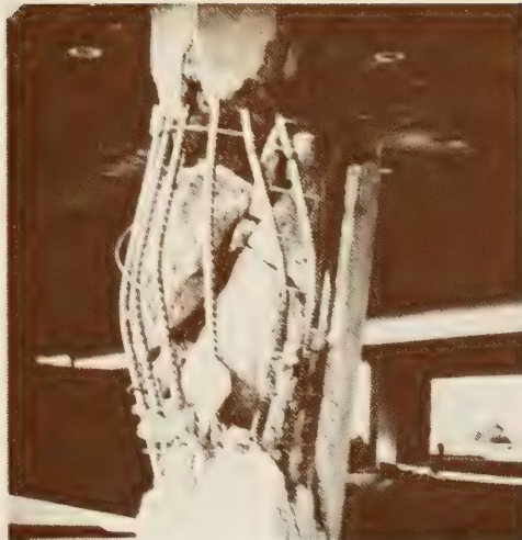
Figure 3.—Failed concrete column core.
